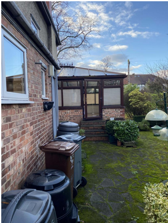
Existing uPVC conservatory to be replaced
