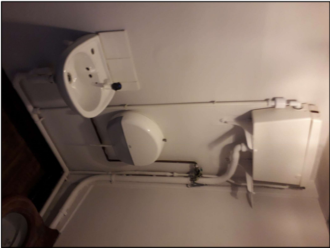
P35 - View of Toilet Area A1/03 - Oversink electric water heater to be installed to provide hot water to wash hand basin.
