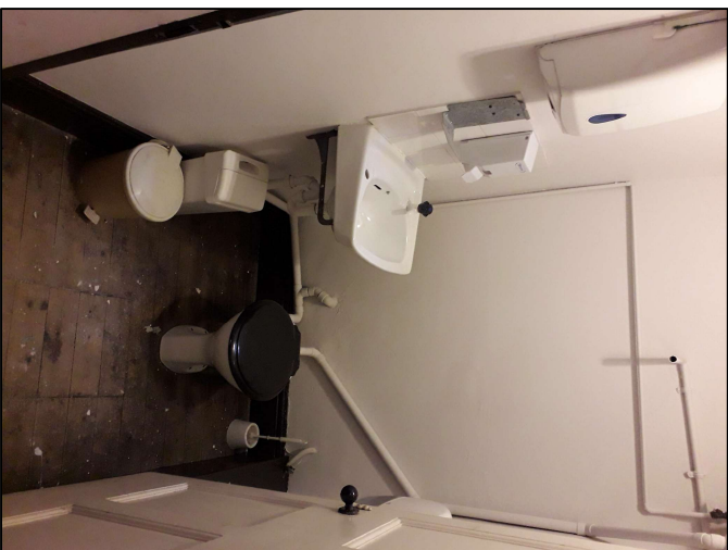
P37 - View of Toilet Area A1/04 - Oversink electric water heater to be installed to provide hot water to wash hand basin.
