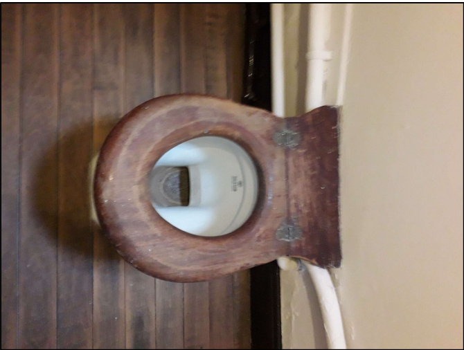
P36 - View of Toilet Area A1/03 - Wooden toilet seat to be repaired and receive 2No. coats of varnish.
