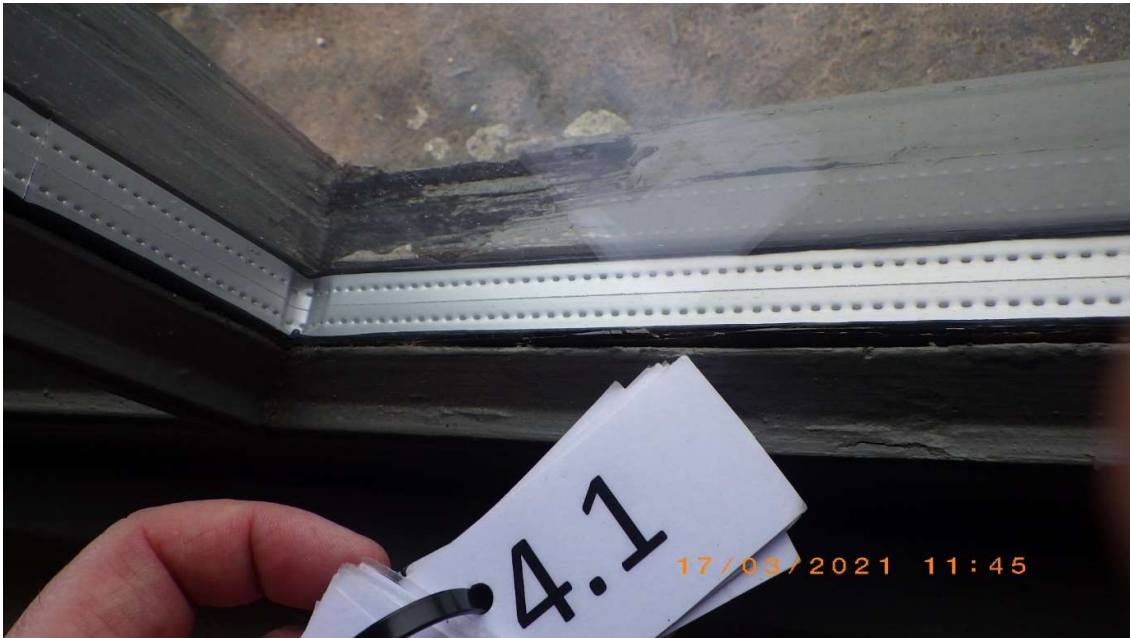
Figure 1 Example of localised decay in window opening light
