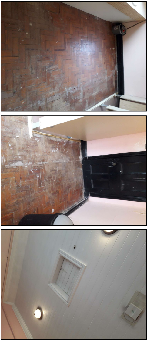
P83 - View of Female W.C. Area A0/31 wood block flooring to be repaired & sanded and sealed.
