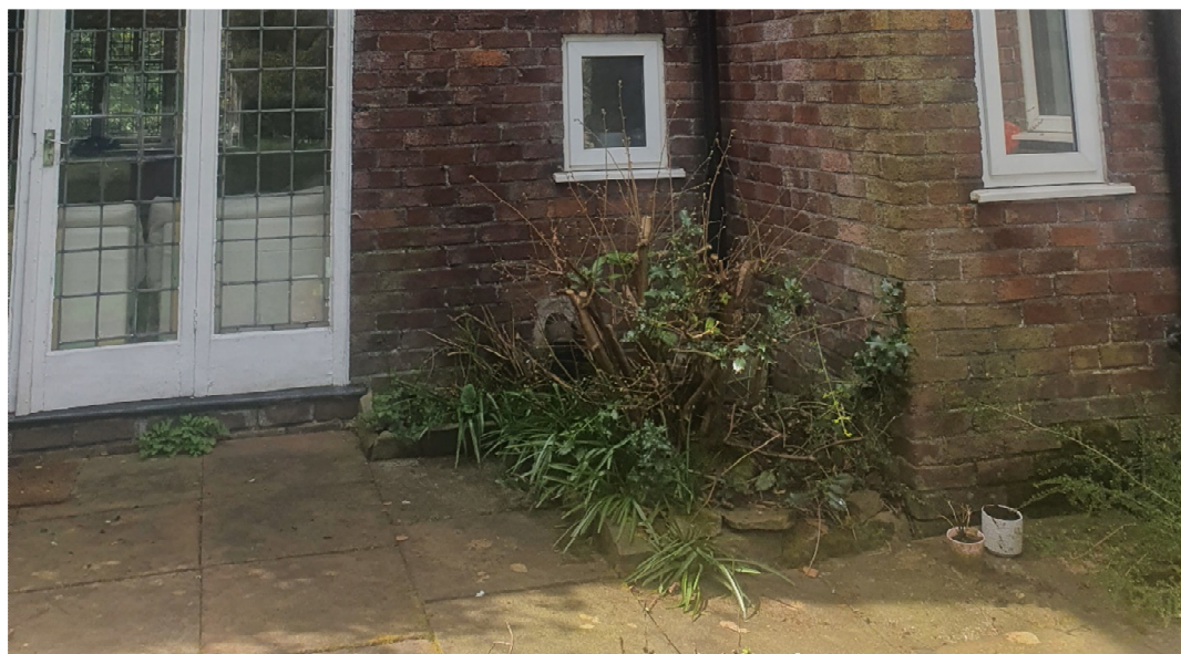
Photo 2: Patio to the rear of the property in relation to the floor level of the property.
