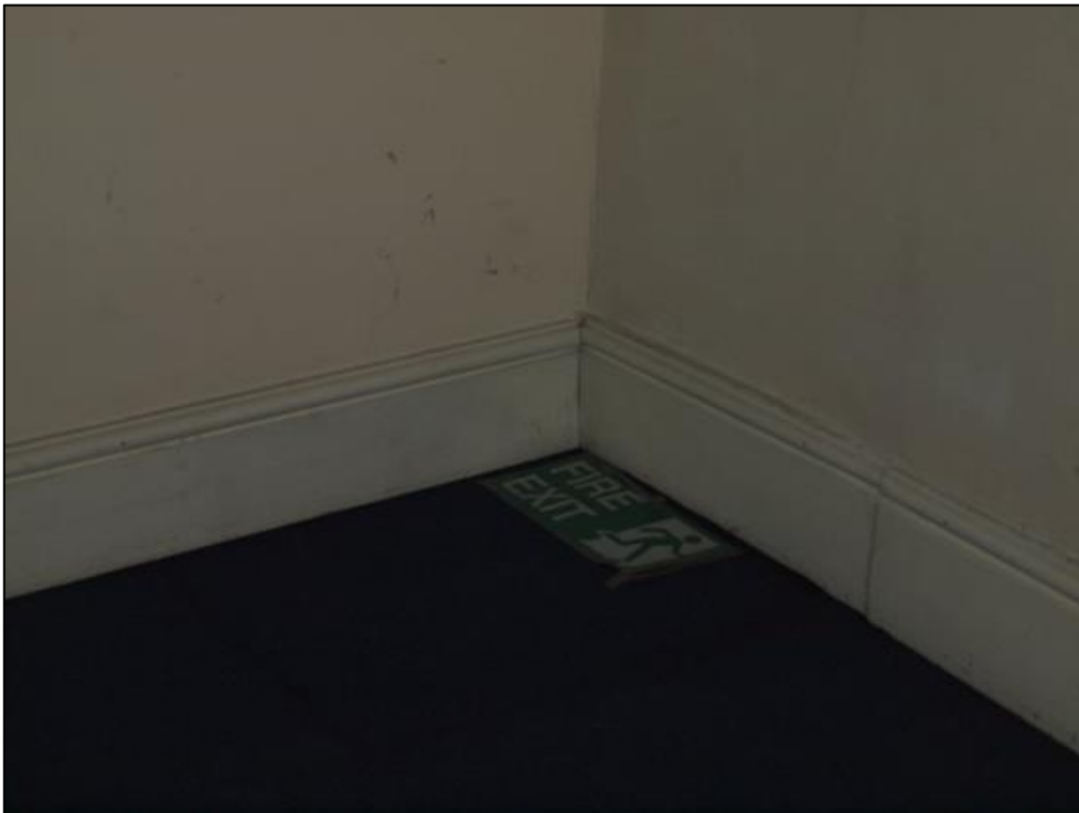
Plate 53: Skirting on top landing
