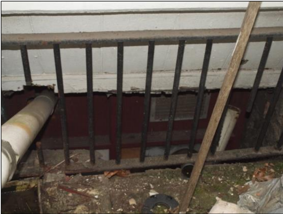
Plate 10: Blocked light well below bay window
