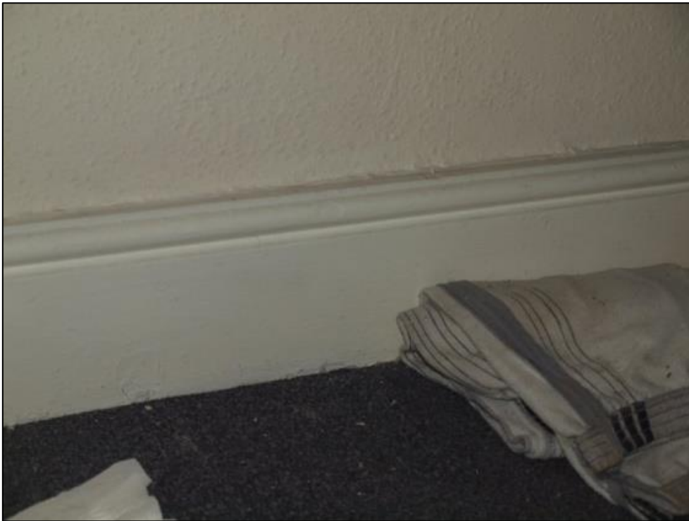
Plate 26: Detail of modern skirting in northwest extension
