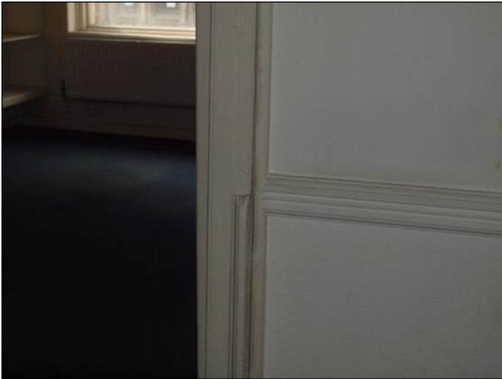
Plate 62: Altered moulding on west side of door surround
