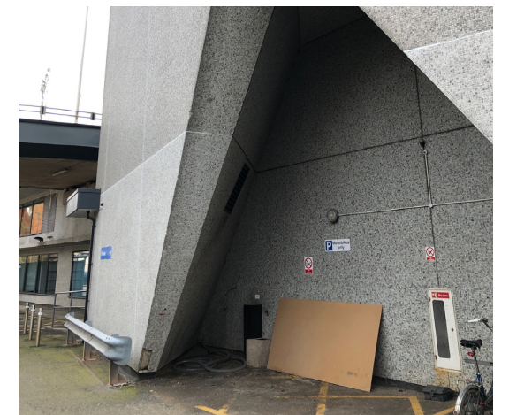
Replacement tiles and white movement joints disrupt the facade uniformity.
