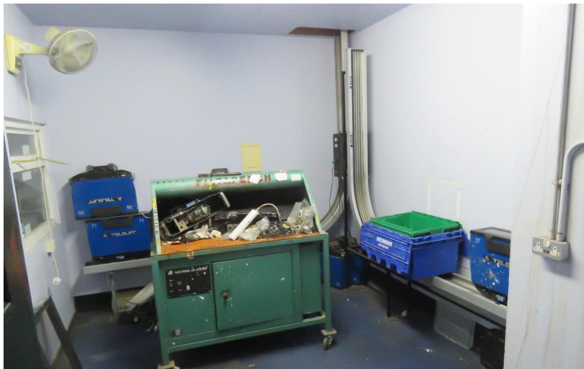
00-15 Detail of the decommissioned Telelift system.
