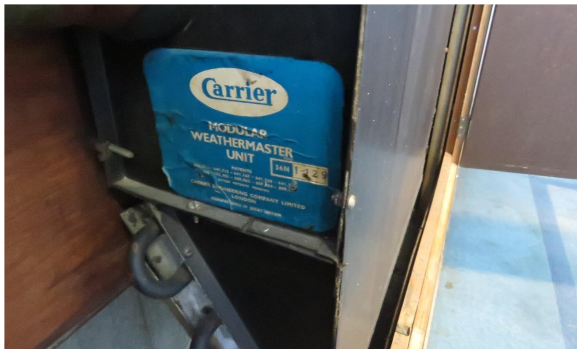
00-09 Detail of the Carrier Company Weathermaster system.
