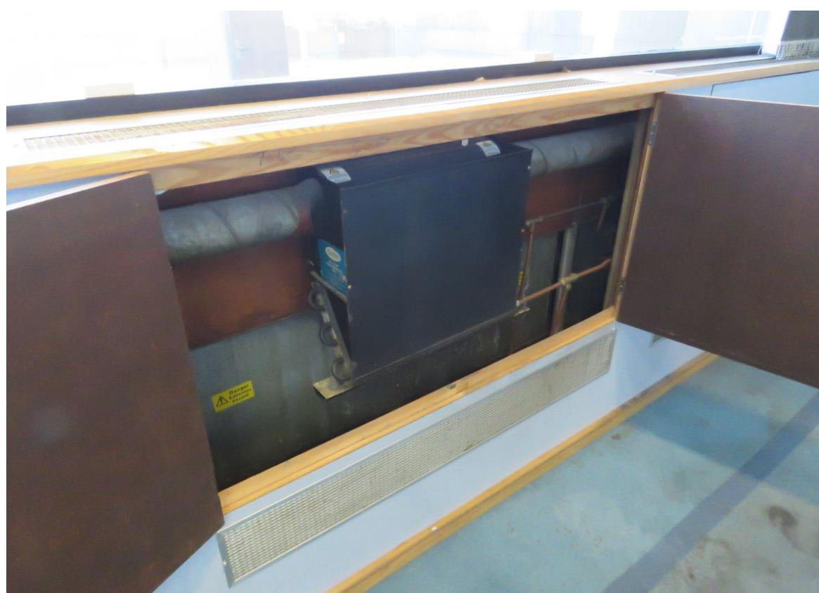
00-08 Detail of the Weathermaster system.
