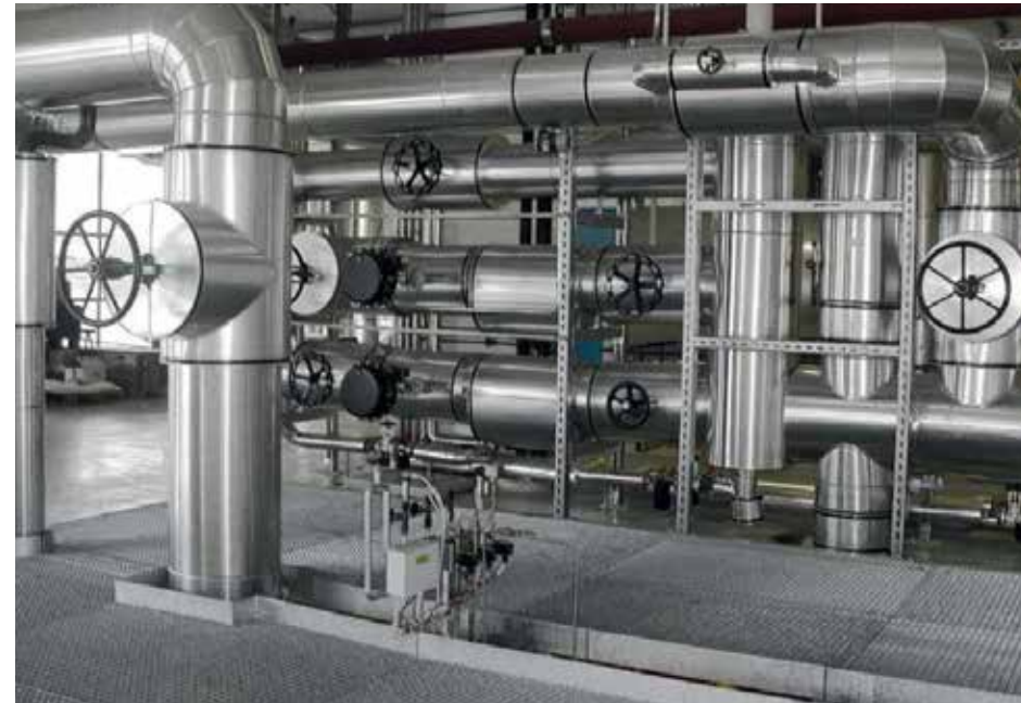
Typical pipework clad in polished metal
