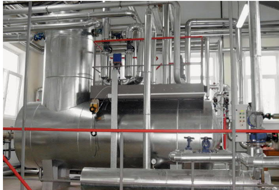
Typical boiler clad in polished metal
