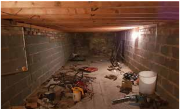
Underneath the 1980s platform - it is unsafe and a further application will be submitted for removal of this non-original structure
