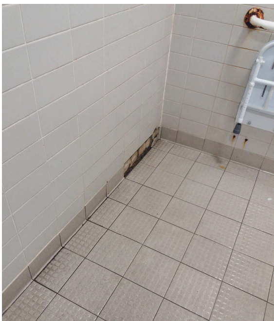
Evidence of internal damage and rusting within changing rooms (image from Nov 2019)
