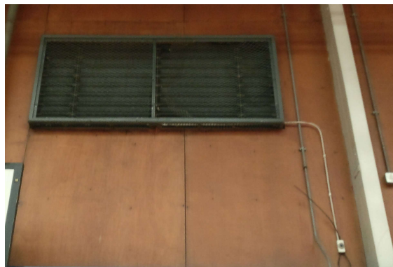
Internal louvre showing evidence of physical damage and missing actuator handle
