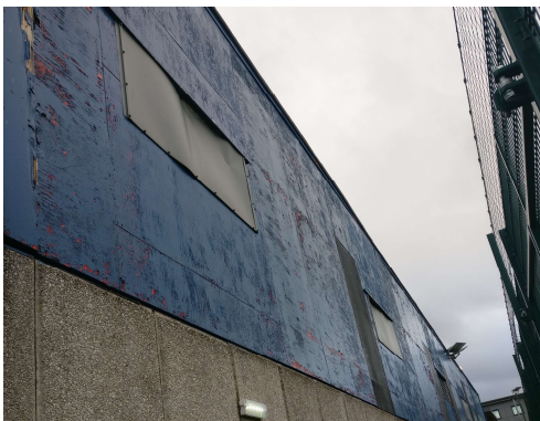
External covered louvre showing evidence of ongoing physical damage
