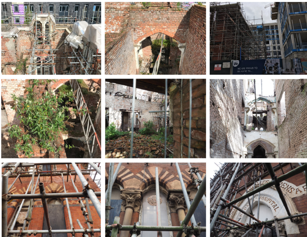
Figure 1: Images showing the condition of Ancoats Dispensary
