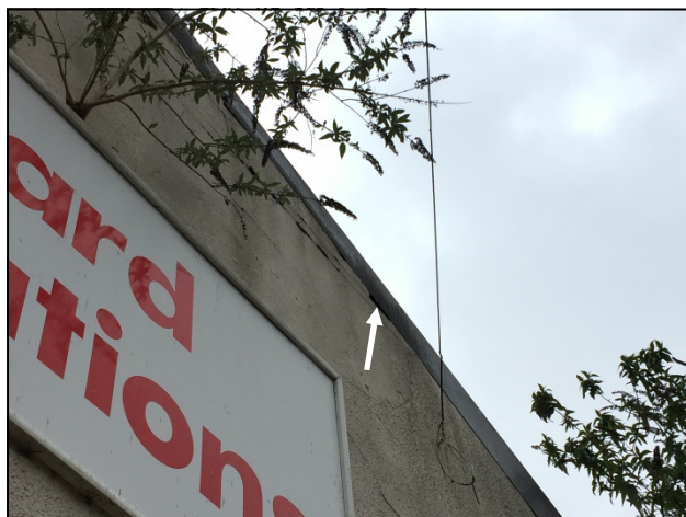
Plate 1 Gaps exist behind fascia boards at gable end
