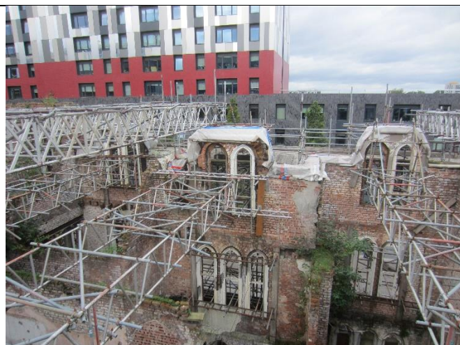
Photo 7: View of the building from above showing exposed condition and absence of a roof covering
