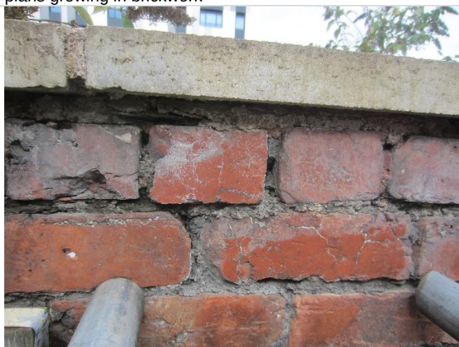
Photo 10: Mortared gaps between brickwork and beneath copings
