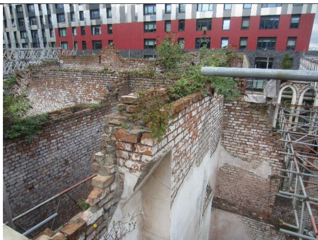
Photo 8: View of the building from above showing exposed condition and absence of a roof covering. Butterfly Bush plants growing in brickwork
