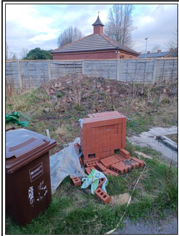
Photo 8, DEBRIS LEVELS ON SITE
