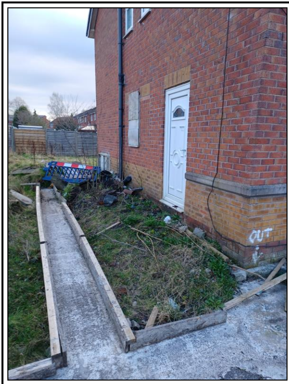
Photo 10, DEBRIS LEVELS ON SITE
