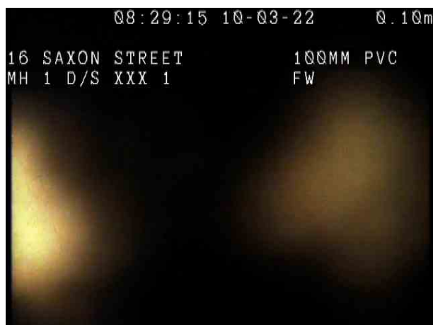
MH 1X_3ee70542-c734-47b2-9bb8-980078789a33_20220310_13 3435_646.jpg, 00:00:12, 0.10 m Settled deposits, fine, 90% cross-sectional area loss
