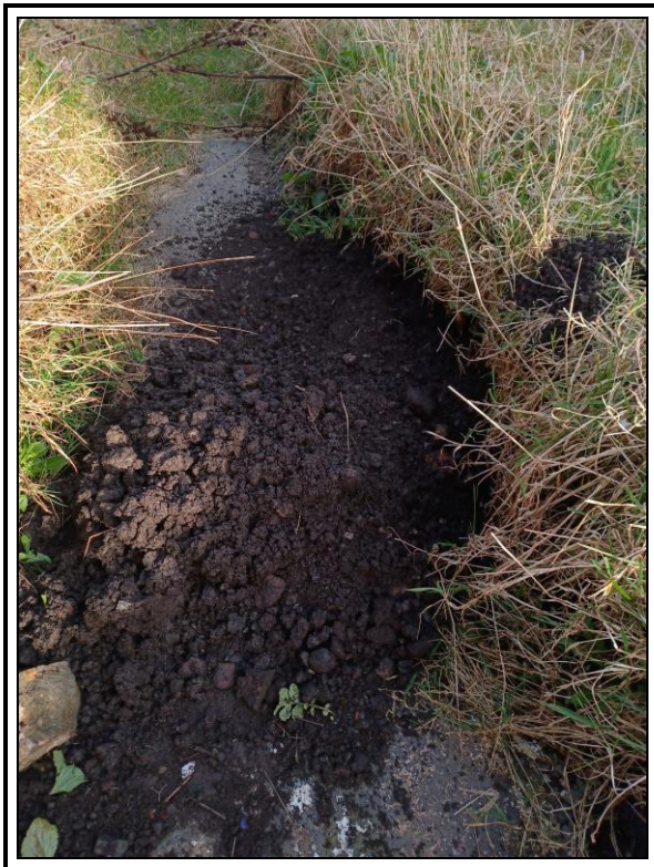
Photo 4, MH 1 SILTED AND AMOUNT REMOVED
