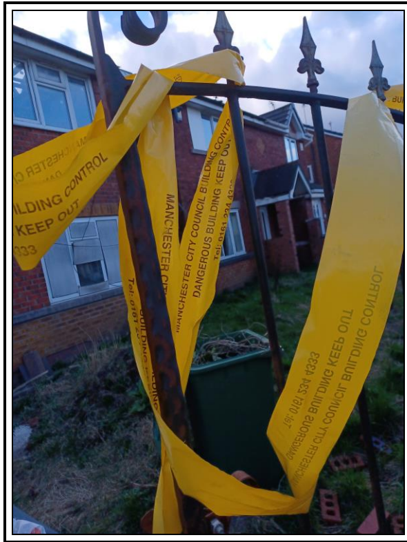
Photo 7, DEBRIS LEVELS ON SITE AND COUNCIL DANGER WARNING TAPE
