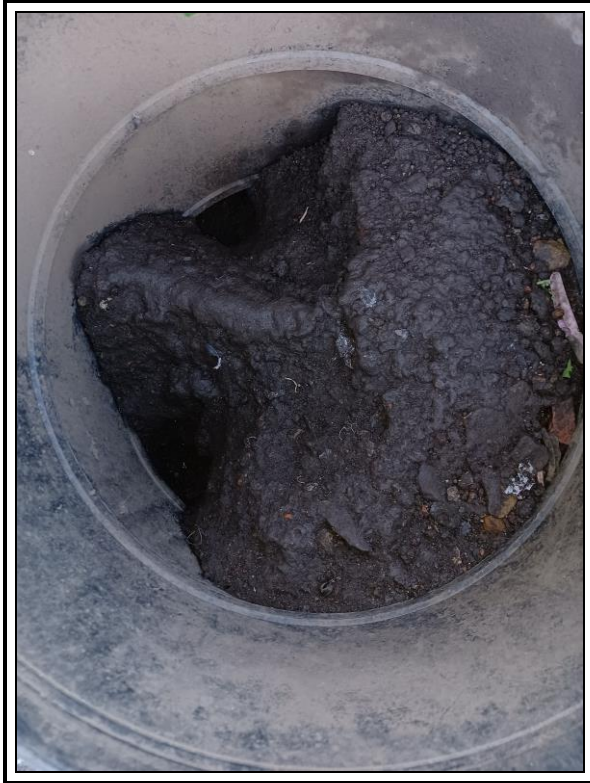
Photo 3, MH 1 SILTED AND AMOUNT REMOVED
