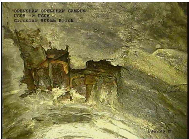
UC05X_3a7e4e4e-80cf-46fa-b935-b415f066d653_20200612_120931_208.jpg, 00:18:36, 104.95 m Missing bricks from 1 o'clock to 2 o'clock
