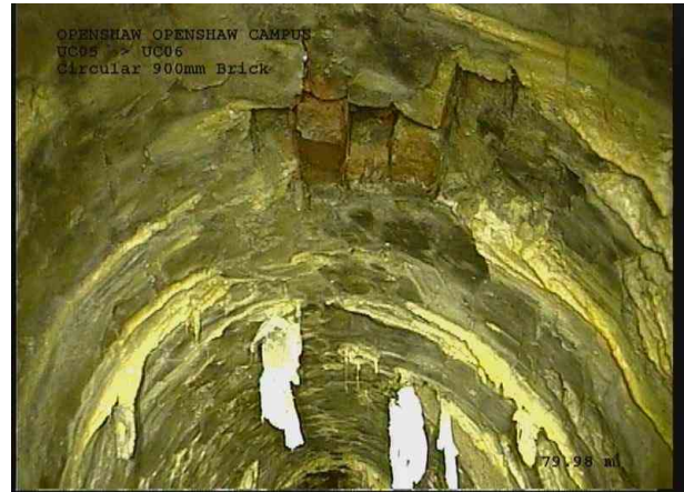
UC05X_4bbd8acb-7a18-400f-8141-a86006ade5ca_20200612_120429_867.jpg, 00:13:50, 79.98 m Missing bricks at 12 o'clock
