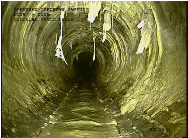
UC05X_f57ceeea-3490-4ac7-894e-edc87a541434_20200612_115413_741.jpg, 00:06:04, 37.55 m Infiltration, dripping from 12 o'clock to 1 o'clock
