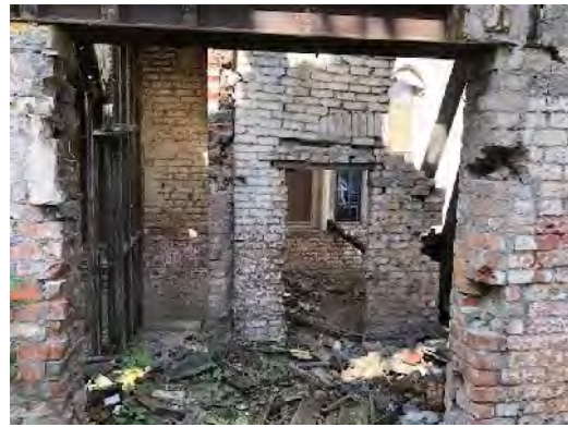
View of the internal structural instabilities
