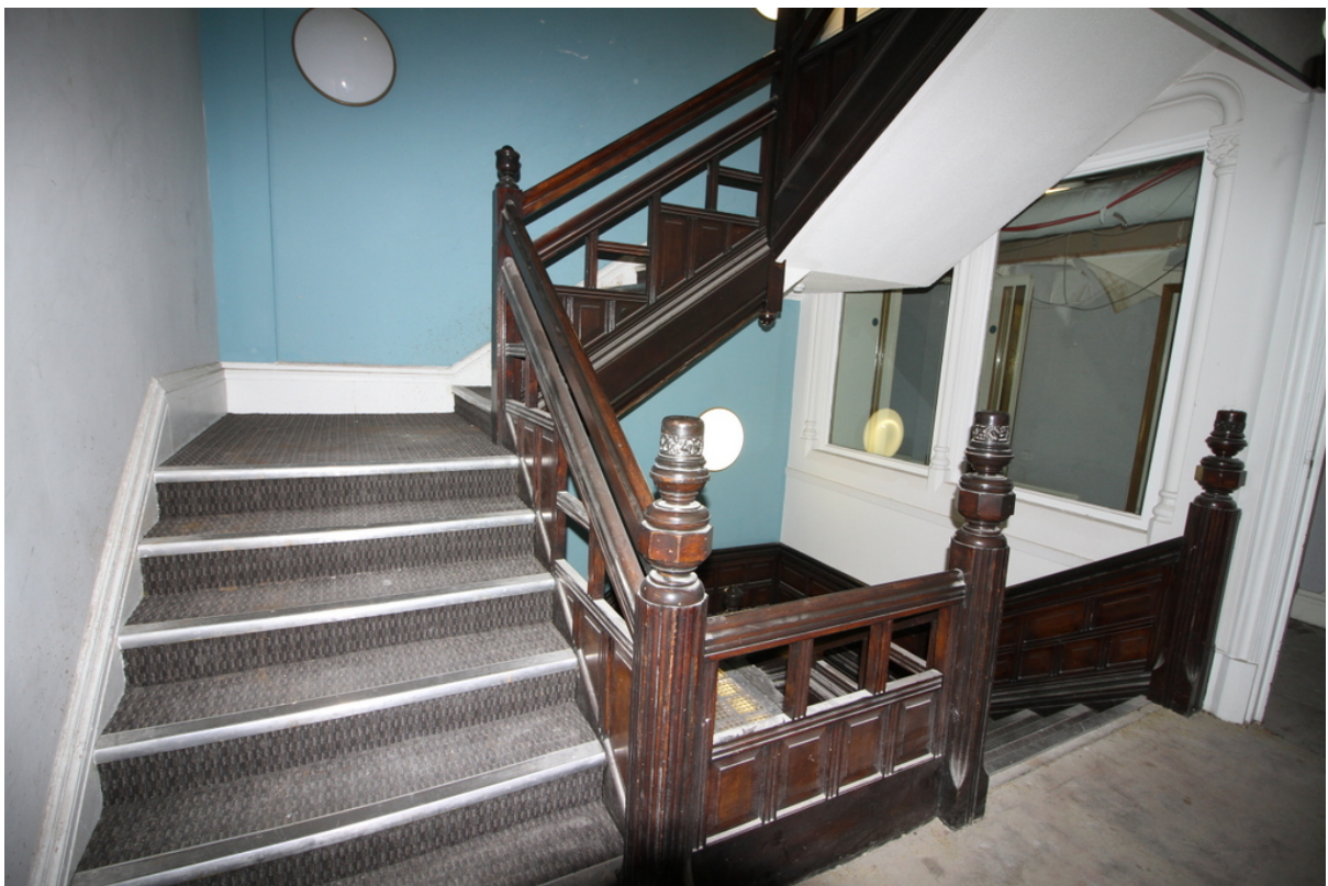
Moulding compromised by later stairwell
