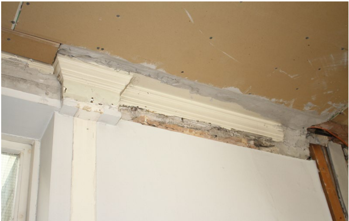
Damaged and missing in various places
