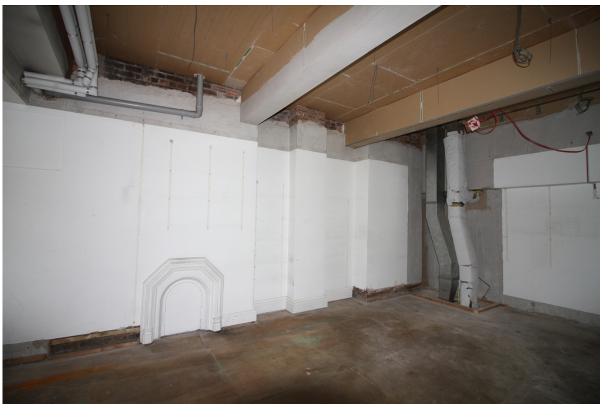
Second floor ceiling in rear room, with scars of original and late ceilings, both removed, and clearly showing modern plaster above the position of the suspended ceiling
