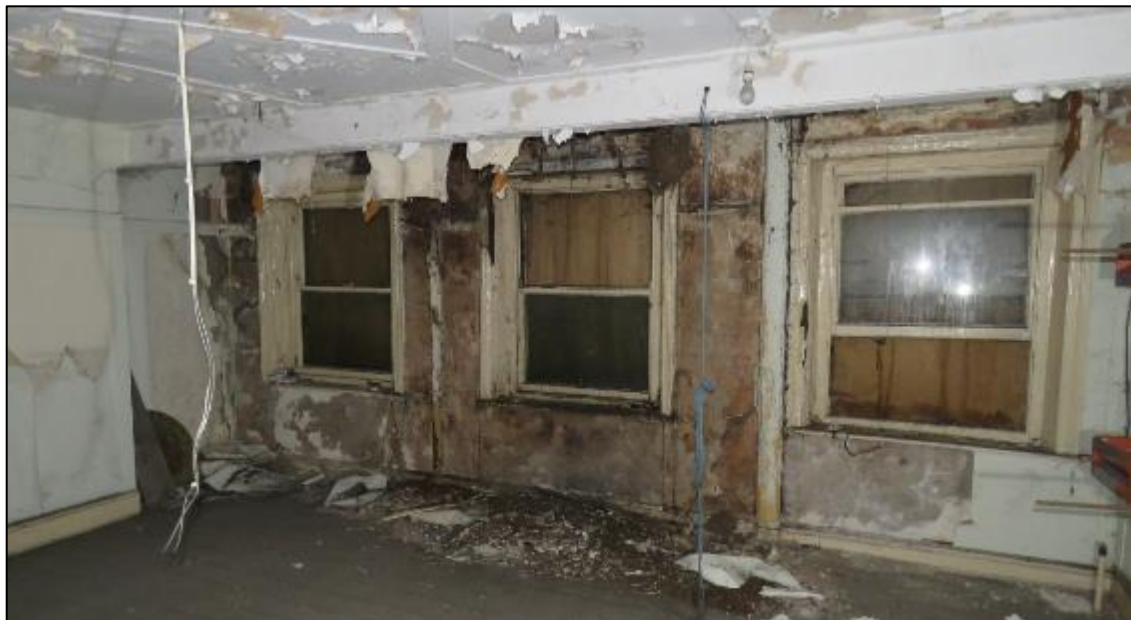
Figure 49. View looking toward Piccadilly (March 2019) showing the surviving sash-windows which retain their original architraves in very poor-condition. The internal walls have been removed to create a single large-space. The interior plaster and decorative details are largely early-C20th.
