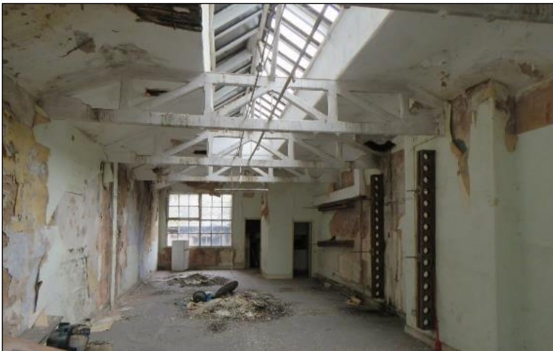
Figure 54. View from the second-floor of the warehouse (March 2019), looking towards Piccadilly. The access to the former dwelling is via the remnants of the original outrigger (top -right of view). The steel clamps/braces have partially supported the flank wall following the demolition of 43-45 Piccadilly.
