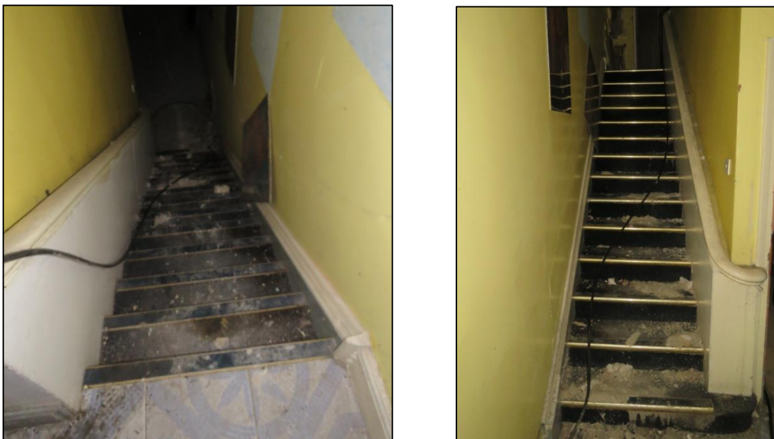
Figure 40b. View of the altered and narrow stairs from Ground to First floor.
