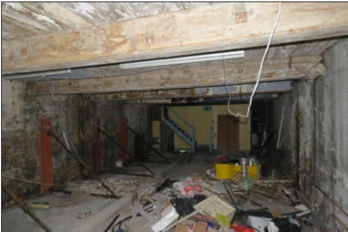
Figure 37. View looking-north toward Back Piccadilly (March 2019) . Note the modern bracing to the west wall resulting from the demolition of the premises at 43-45 Piccadilly.
