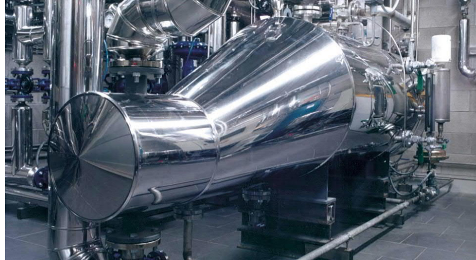
Figure 7-7 - typical steam equipment - polished metal cladding - example
