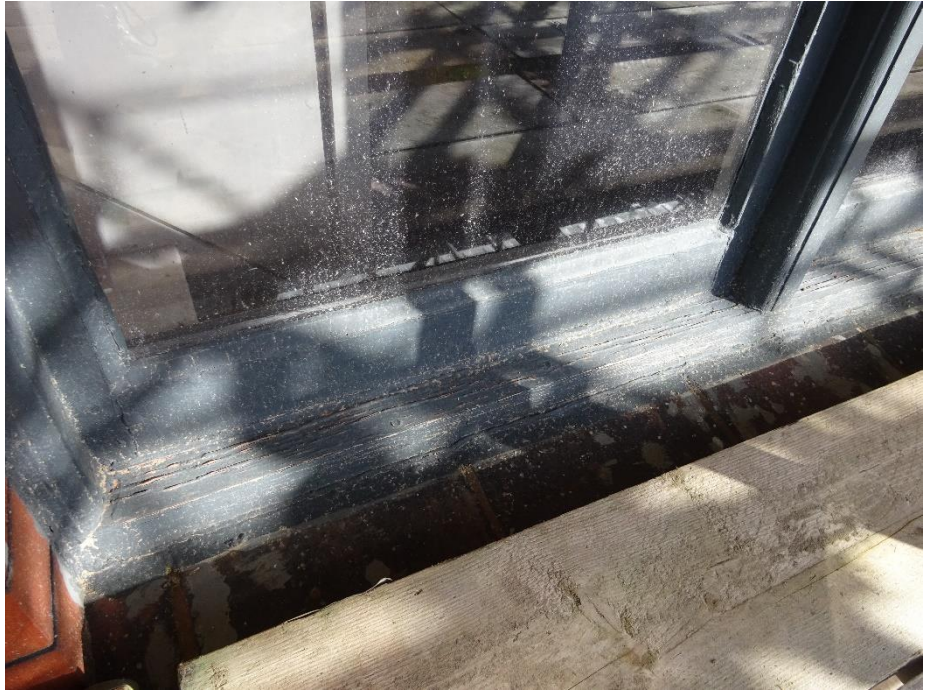
View of weathered and cracking paint to windows to South elevation.
