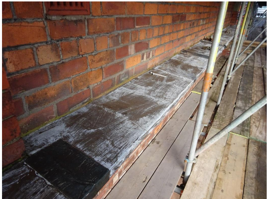
View of patch repairs and a crack to the lead projecting cornice to the East elevation.
