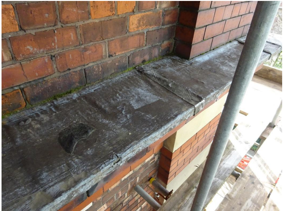
View of damage to the lead projecting cornice to the West elevation.
