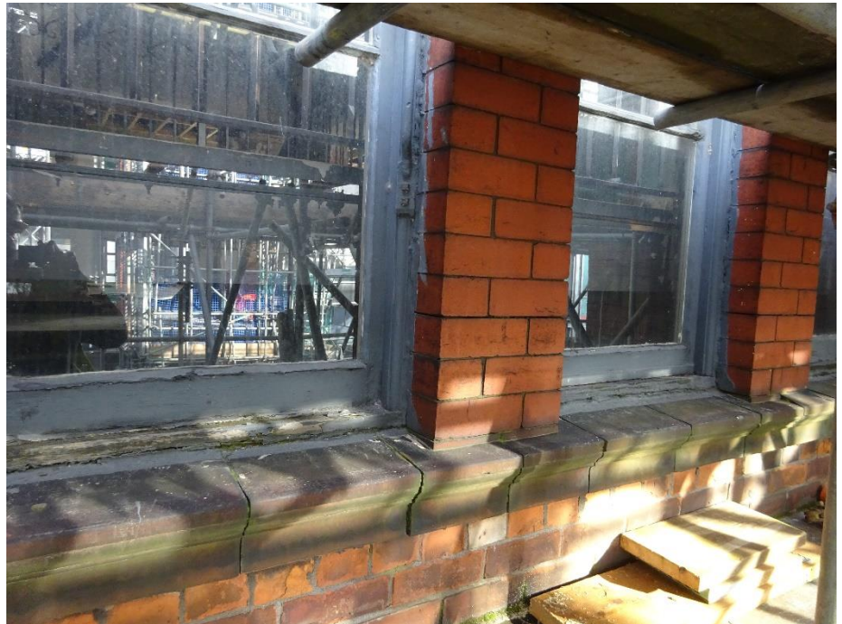
View of rotten window cills, West elevation, 3 rd floor level.
