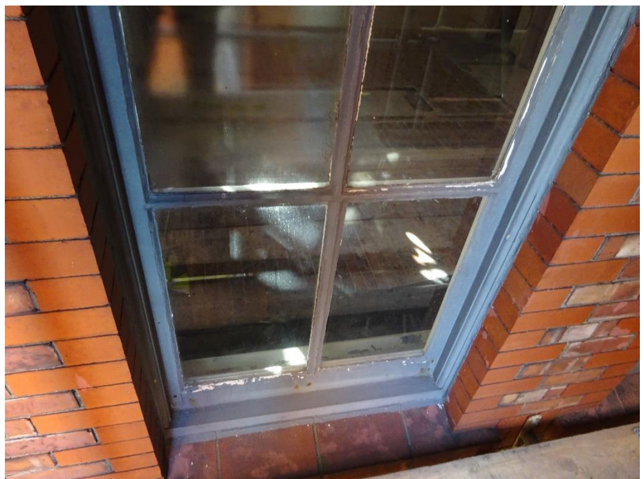
View of peeling paint to 2 nd floor window, North elevation.
