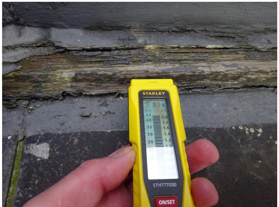
Moisture reading or damp/rotten windows to West elevation, 3 rd floor level.
