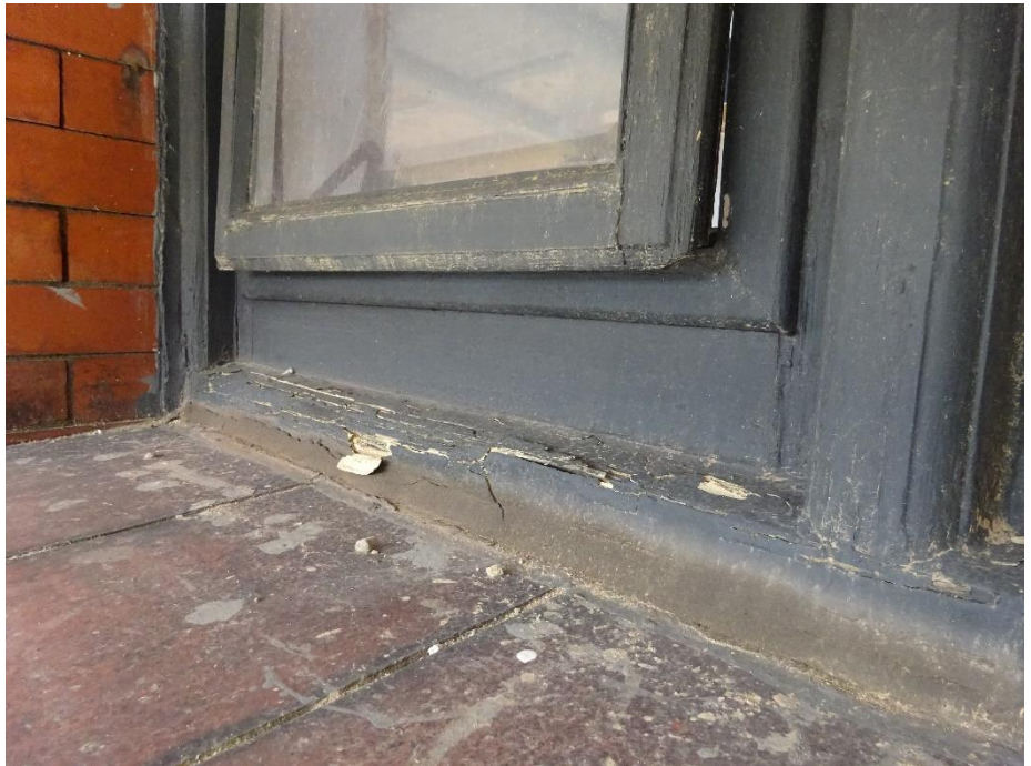
View of peeling paint to 1st floor window, south elevation.
