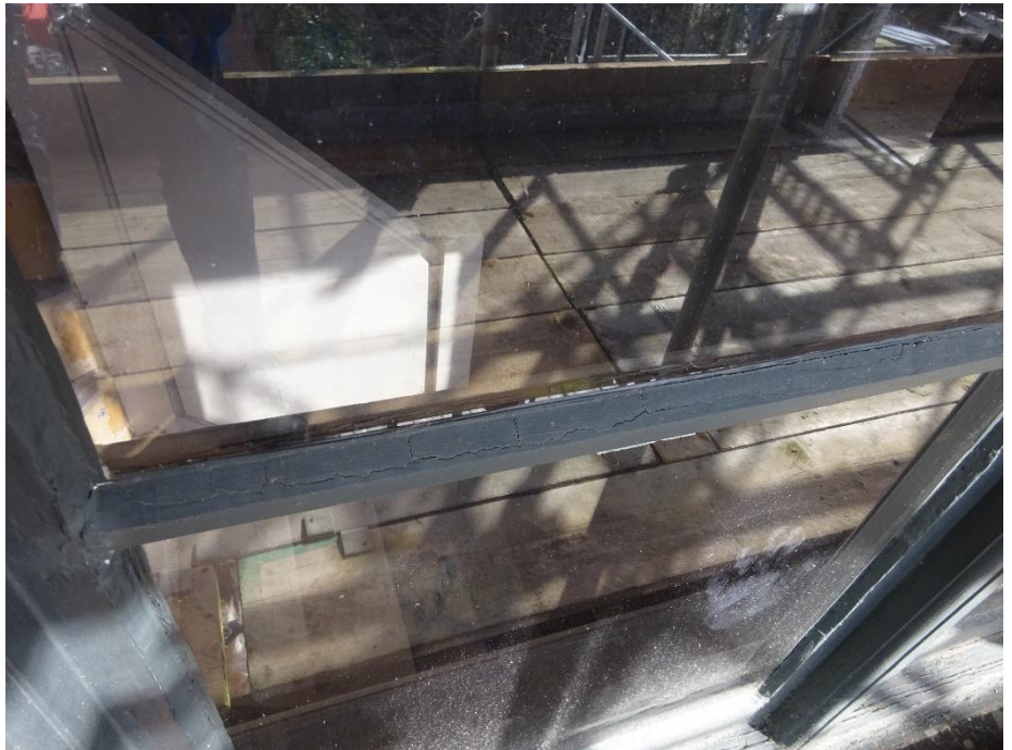
View of brittle and cracked paint and timber to window to South elevation.
