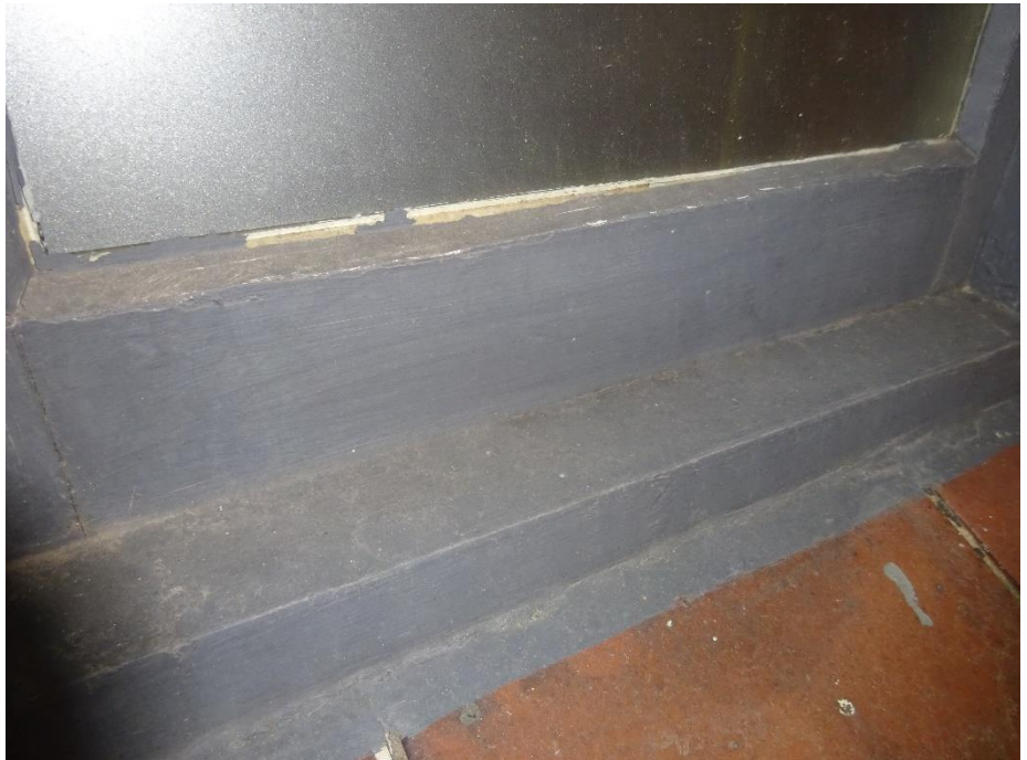
View of peeling paint to ground floor window, North elevation.
