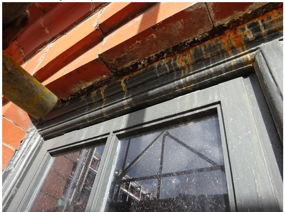
View of heavily soiled windows and repointing/new sealant required to window on South elevation.
