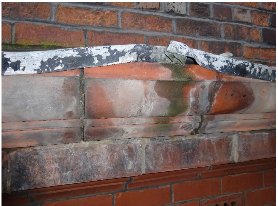
View of a damaged lead projecting cornice to the East elevation.
