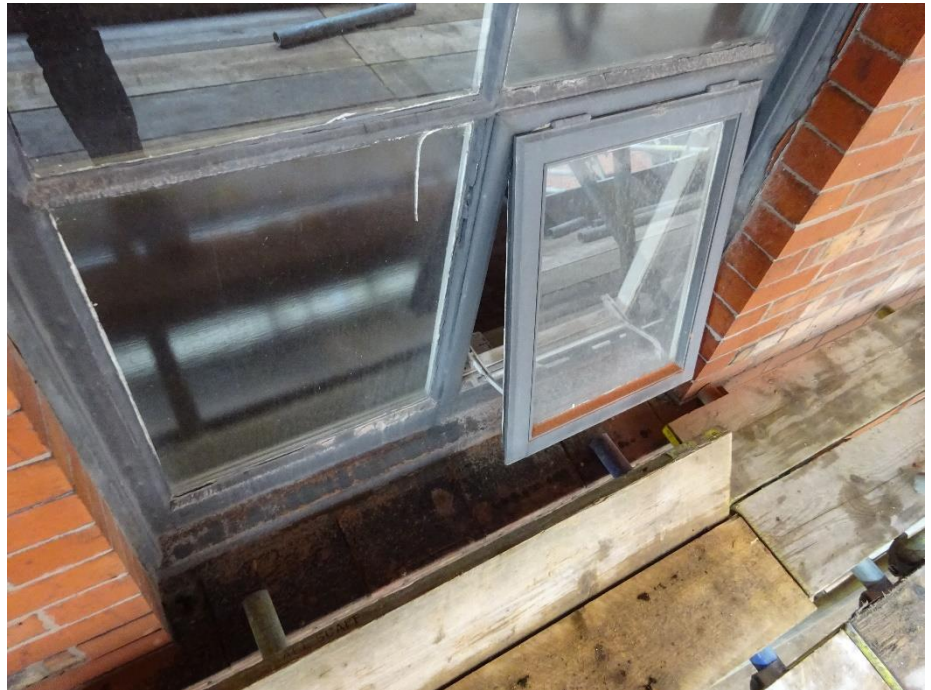
View of peeling paint to 2 nd floor window, East elevation.
