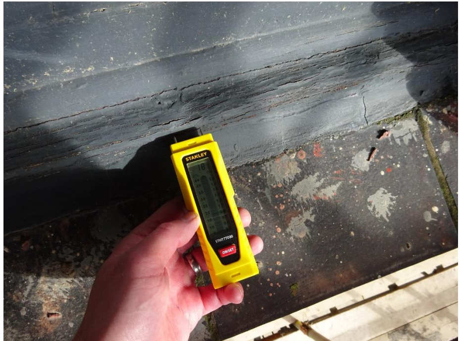
Moisture reading or damp/rotten windows to South elevation, 2 nd floor level.
