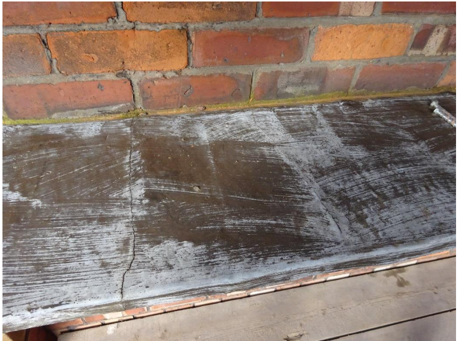
View of crack in lead projecting cornice, East elevation.
