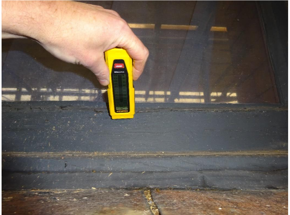
Moisture reading or damp/rotten windows to South elevation, ground floor.
