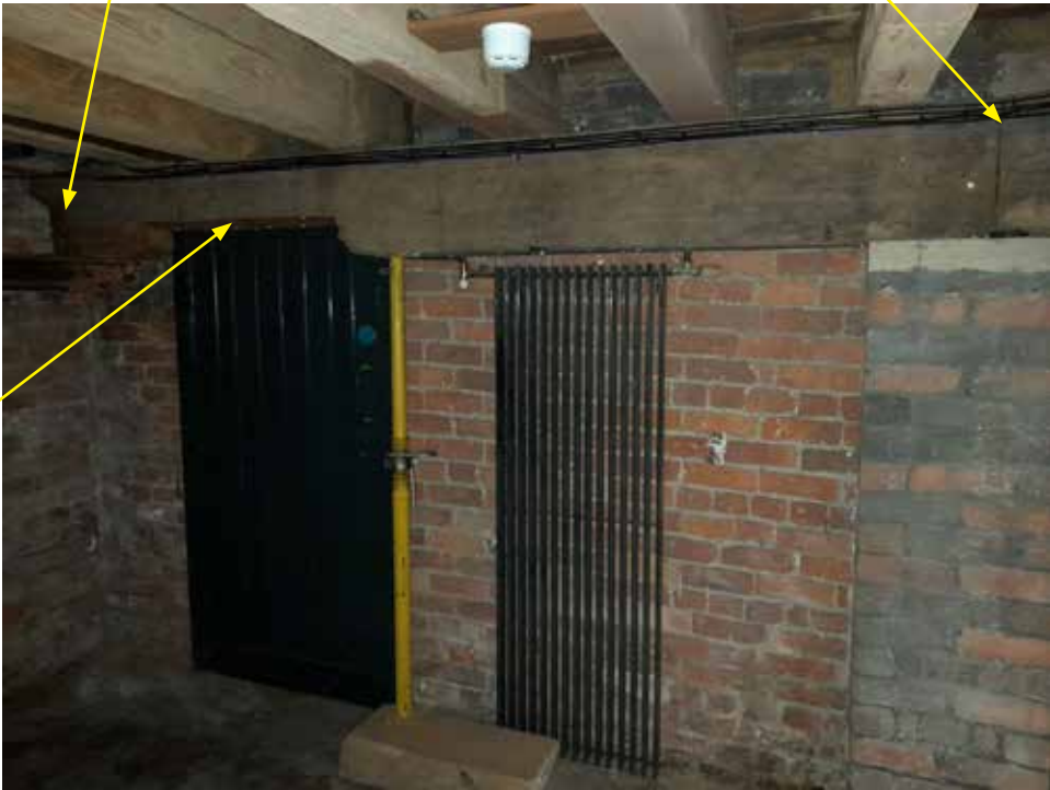
Photograph of existing beam in Bay 1 Basement. The decayed beam end is visible to the left hand side, the existing joint showing the extent of the existing beam is visible to the right hand side.
