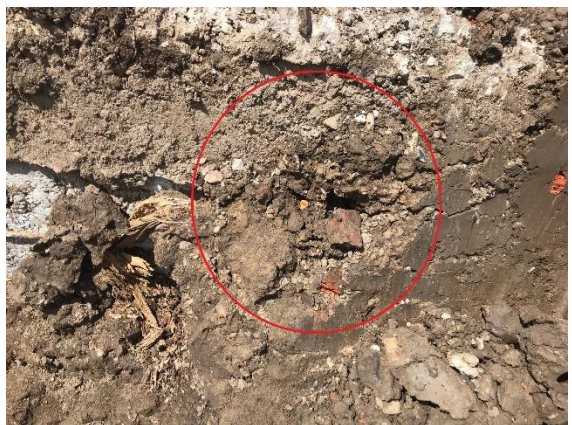
Evidence of rhizome being present in ground that is currently supporting the existing manhole/associated pipe structures.
