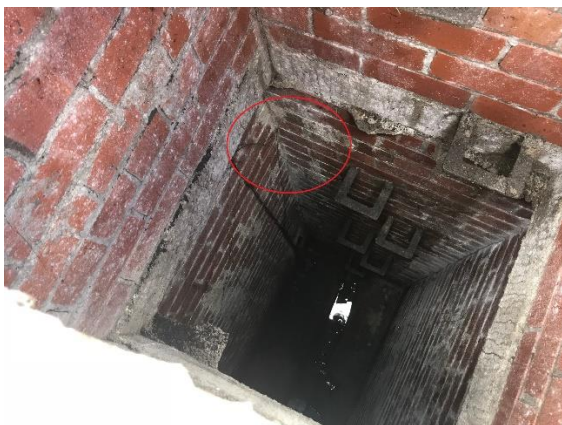
Evidence of rhizome being present within manhole structure.
