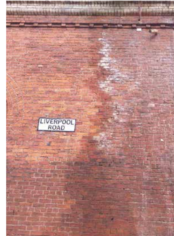
Efflorescence on exterior south facade
