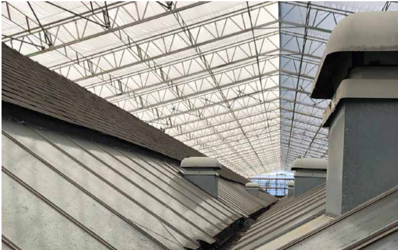
View of the central valley roof and defunct ventilation units cutting through the rooflights
