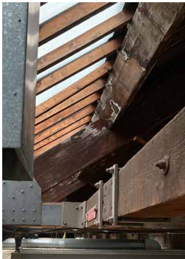
Water damage to existing timber roof structure
