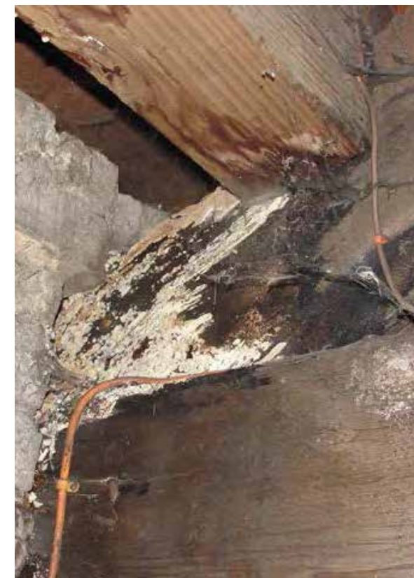
Rotting timber where trusses meet masonry
