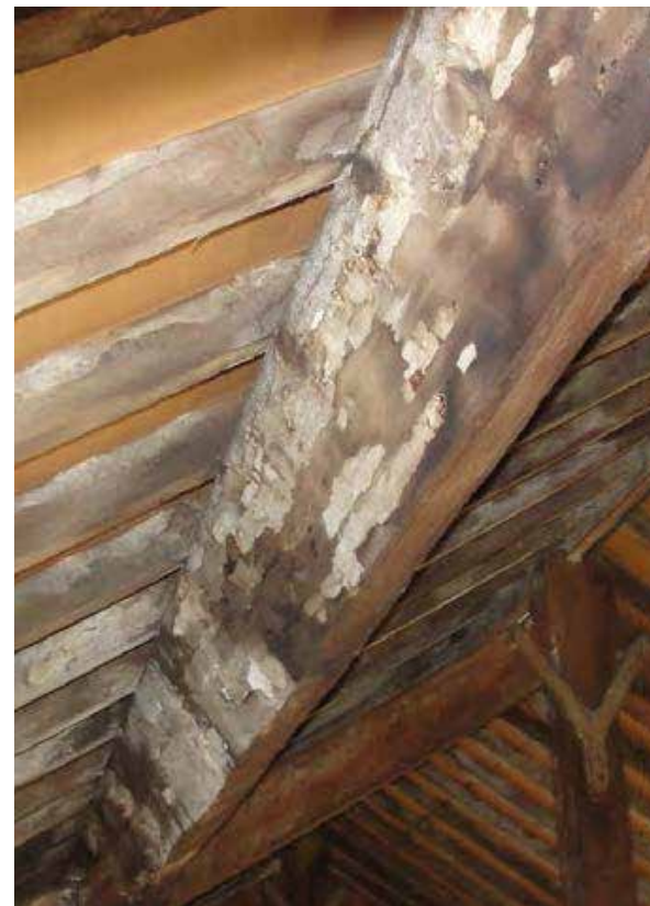
Water damage to existing timber roof structure
