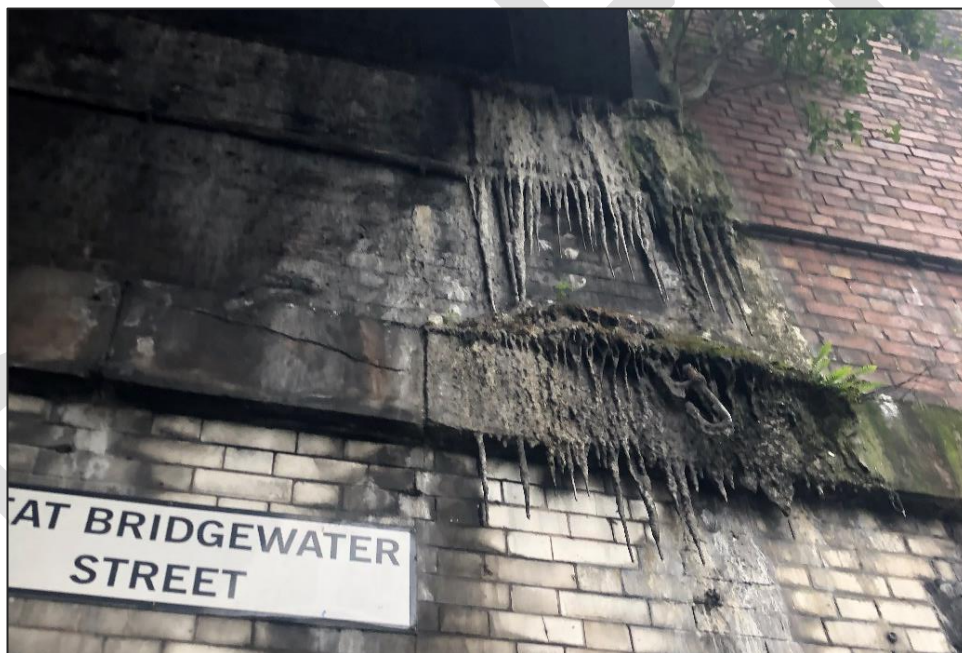
Figure 7: Example of stonework in poor condition due to water ingress.
