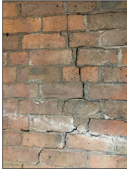
Figure 11: Example of a large crack in existing brick wall (west side).
