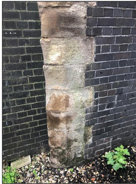
Figure 6: Example of stone quoins, external withlight erosion to the surface.
