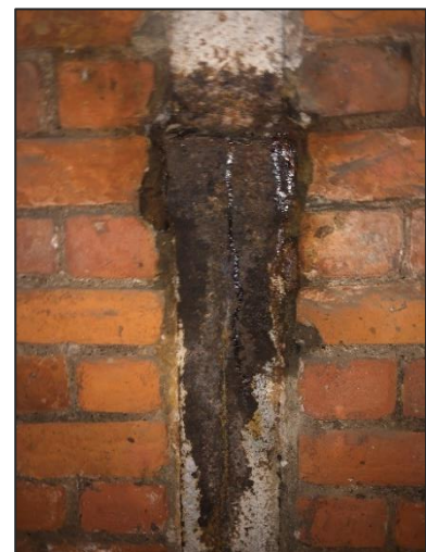
Figure 12 (right): Example of cast iron pipe set into brickwork. Where replacement is required, new pipes should be like-for-like (cast iron).
