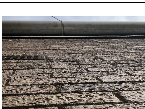
Photo 12: Weatherboard not flush on west side. Does not lead anywhere.
