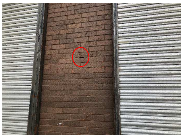
Photo 11: Hole in brickwork on west wall, does not lead anywhere.
