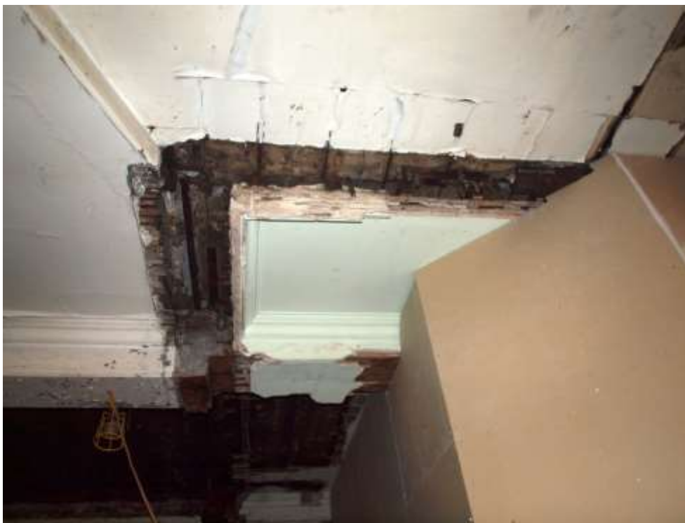
Plate 62: Remains of plaster cornice
