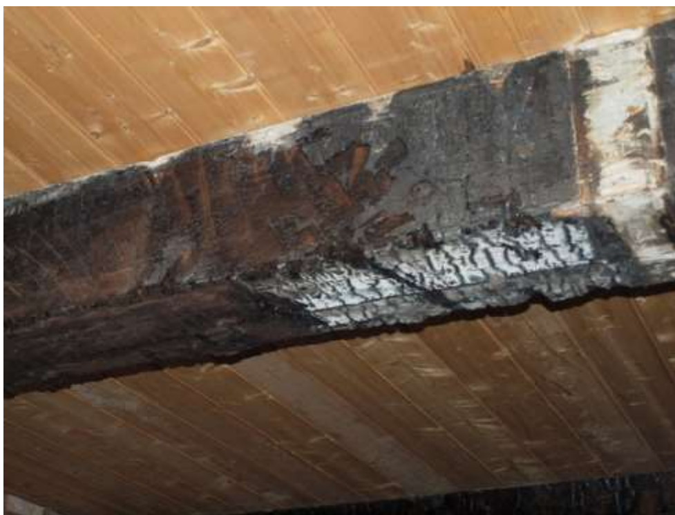
Plate 79: Detail of fire damaged beam
