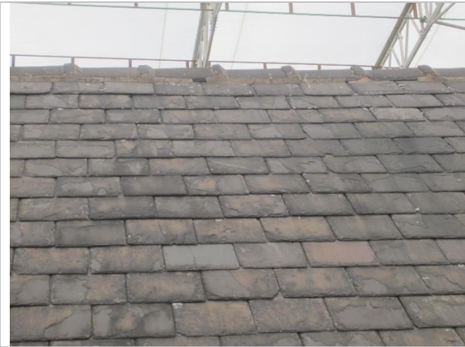
Photo 7: Minor gaps beneath ridge copings
