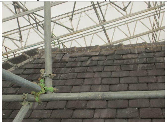
Photo 6: Minor gaps beneath ridge copings
