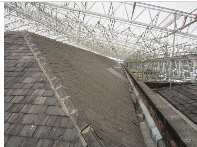
Photo 9: Minor gaps beneath ridge copings
