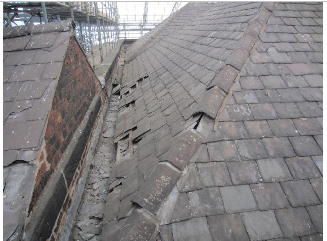
Photo 8: Minor gaps beneath ridge copings and between slates and the board lining
