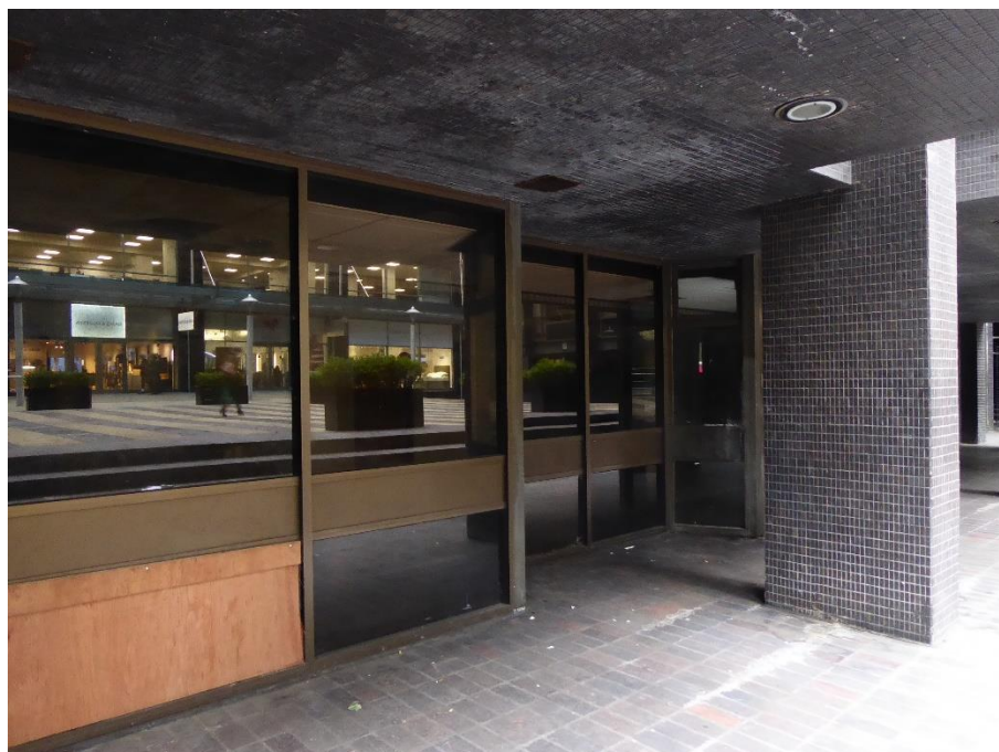
Figure 9: lower level of north elevation where paint finishes appear distinctly different from west facing windows of east elevation (figure 9)
