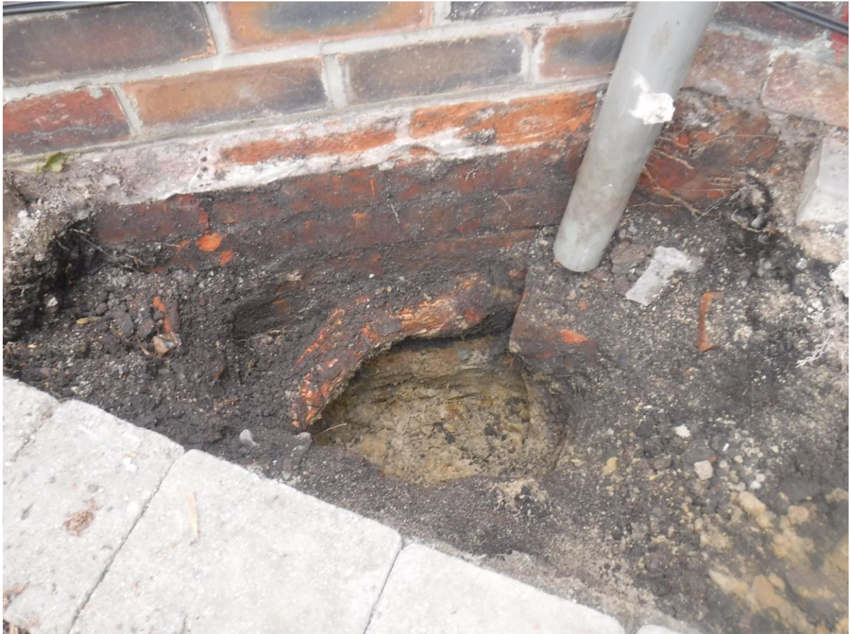
Trial pit – large tree root passing through the wall of the bay window. Base of hole at foundation depth.
