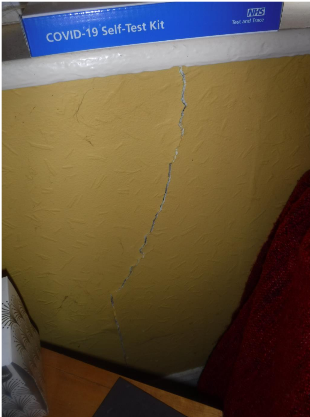
Cracking below the bay window (right hand side). Noted in 2019 report, but may have got worst.
