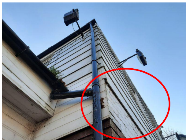
Plate 4.5: Missing Cladding to North
