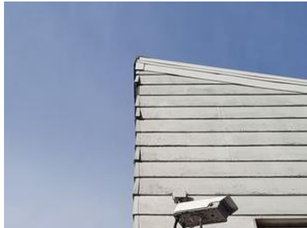
Plate 4.4: Lifted and Missing Cladding Joints
