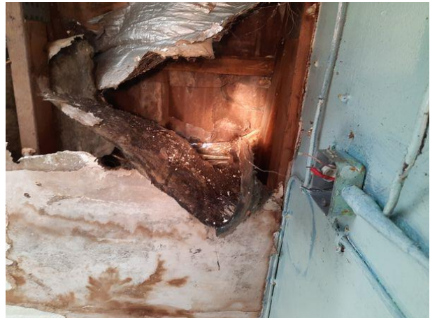
Plate 4.11: Broken Ceiling Board in Southern Toilet Block (Section 1)
