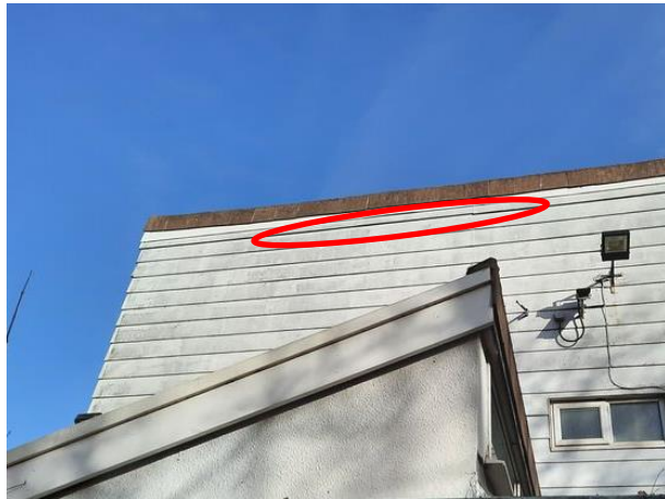
Plate 4.3: Gap Between Cladding
