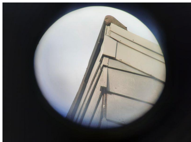
Plate 4.6: Gap Beneath Overhanging Tile
