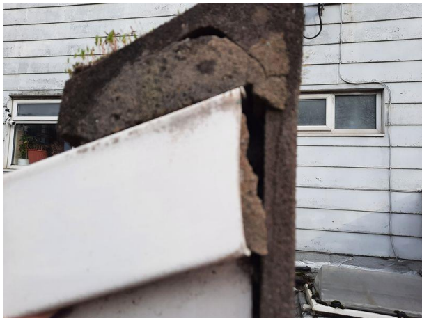
Plate 4.1: Gap in Mortar Below Overhanging Ridge Tile
