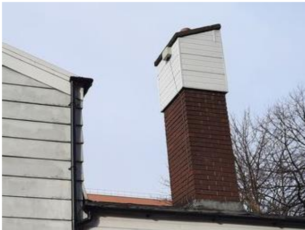
Plate 4.9: Gap Under Chimney Cladding
