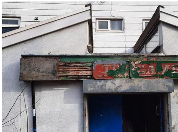
Plate 4.2: Damage to Panelling of Pub Sign on West Elevation of Section 1.
