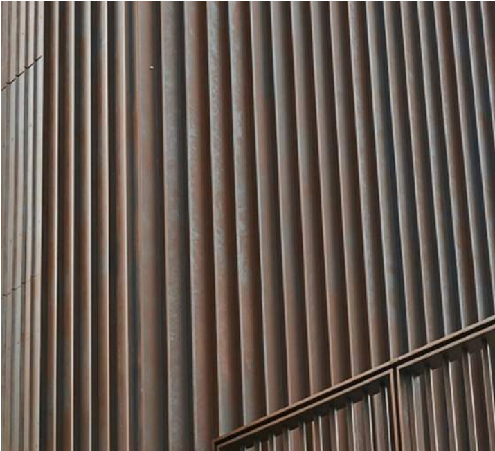
Illustrates subtle changes in colour and tone adding visual interest. Colour to complement but be distinct from brickwork above
