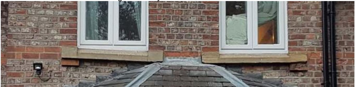
First floor window lintels over the ground floor bay window roof, showing obvious signs of drop and movement
