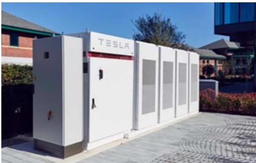
Figure 3.5 An image of external mounted battery for future flexibility
