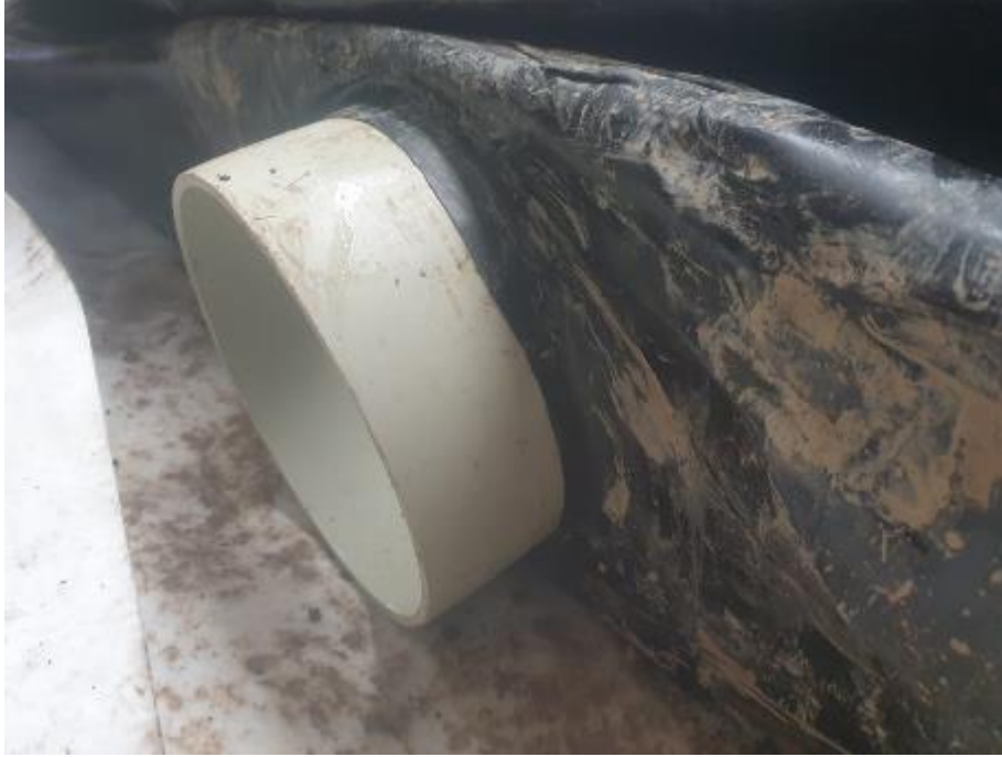
04FEB21 225mm Inlet Connection at Tank Invert Level – Outside View
