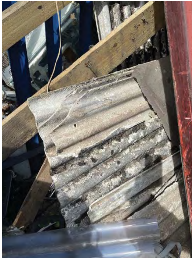
14 Asbestos sheeting at northern boundary of study site.
