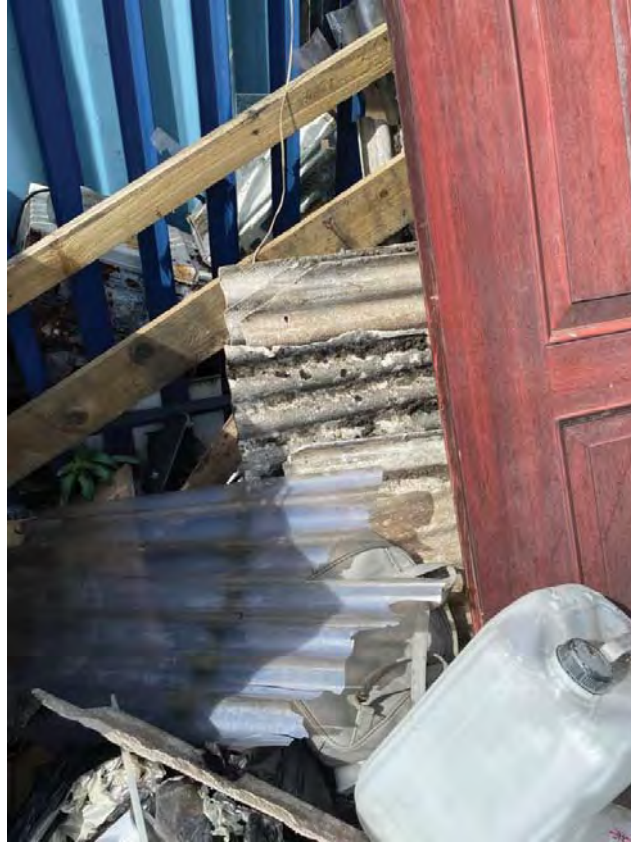
13 Asbestos sheeting at northern boundary of study site.
