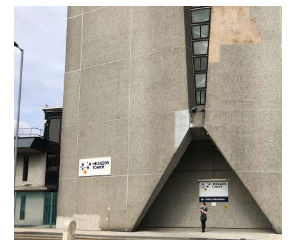
'Bookend' elevation where new tiles and white joints are apparent.
