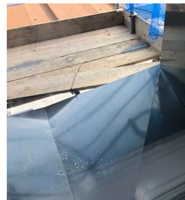
Overcladding in sheet metal (test) on site to 1 window: not a long term solution or cost effective sepcification / installaion method for the entire building
