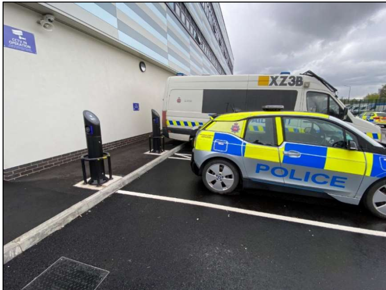
Figure 3.3 – Electric Vehicle (EV) Charging Bollards
