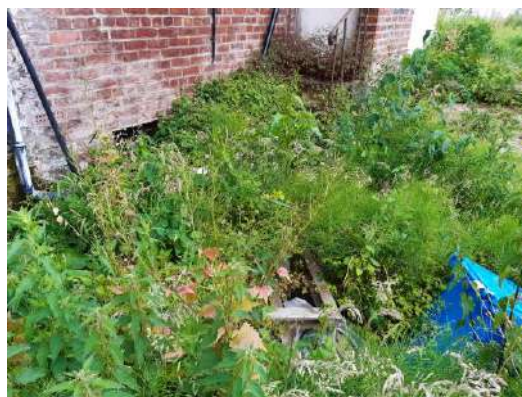
View of possible area of sunken ground immediately to the north of 309 Dickenson Road
