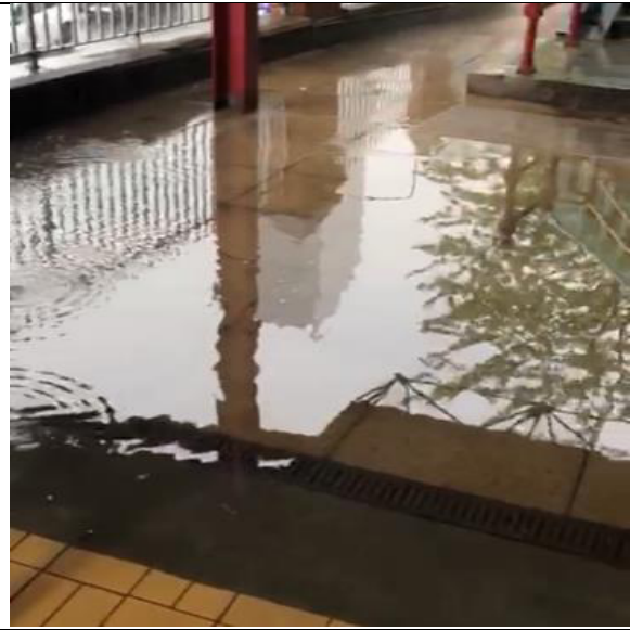
Historic flooding, aco drain not adequate
