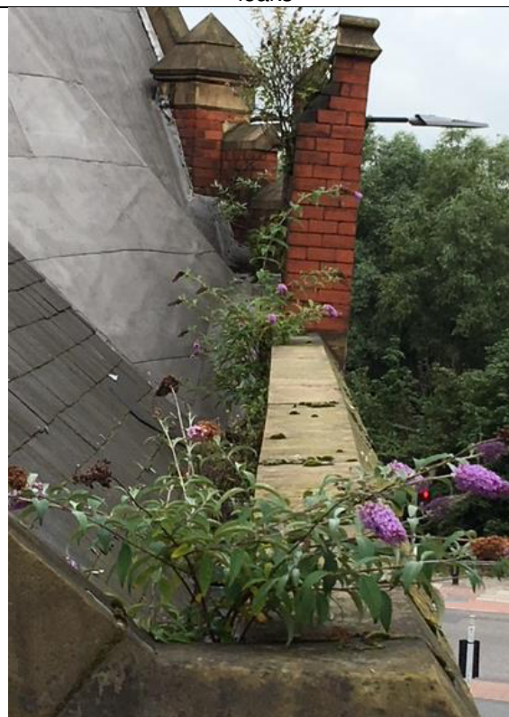
Buddleia through the parapet. Possibly damaging stonework
