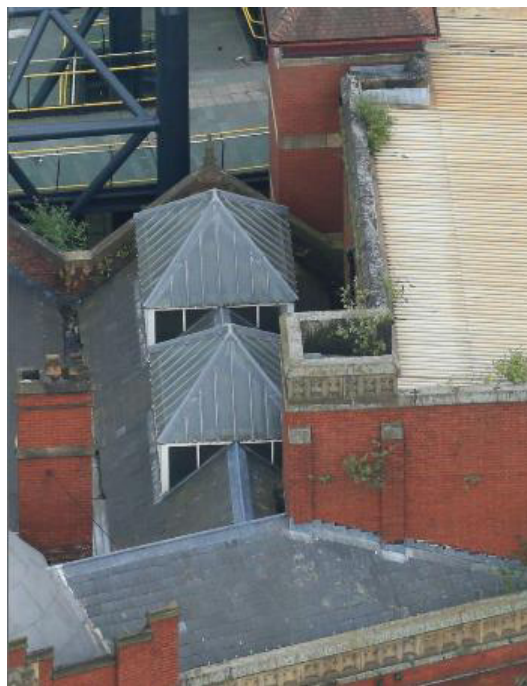
Timbers and flashings over glazed roof to be inspected
