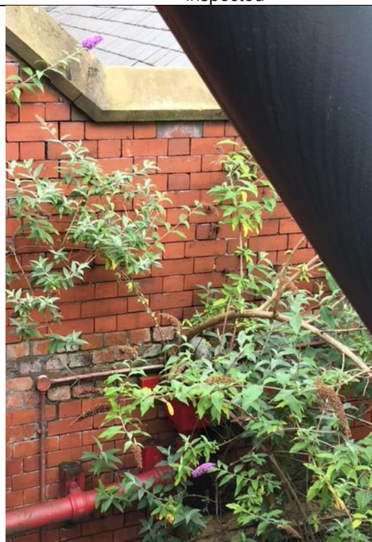
Overgrown vegetation causing damage to brickwork and hopper
