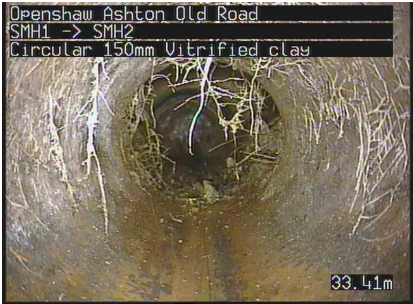
SMH1X_c4a317ae-44a0-4e5f-b158-8d964b1a9f82_20210415_104803_901.jpg, 00:03:50, 33.35 m Roots, tap at joint
