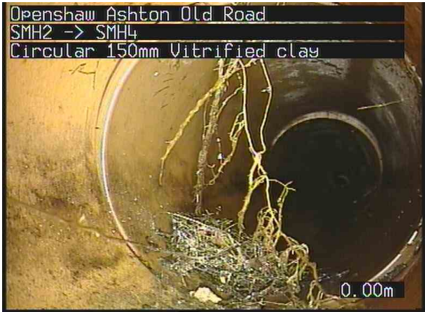
SMH2X_ee43484f-e7f7-473d-87f7-d22fa0666fb5_20210415_112957_740.jpg, 00:00:08, 0.00 m Roots, tap at joint
