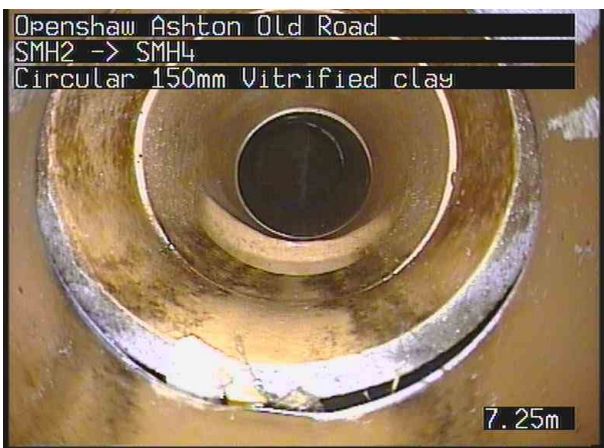
SMH2X_9c6d7cf7-3c68-4f82-b8cb-05fd4beaf2af_20210415_113158_400.jpg, 00:02:00, 7.25 m Joint displaced, medium
