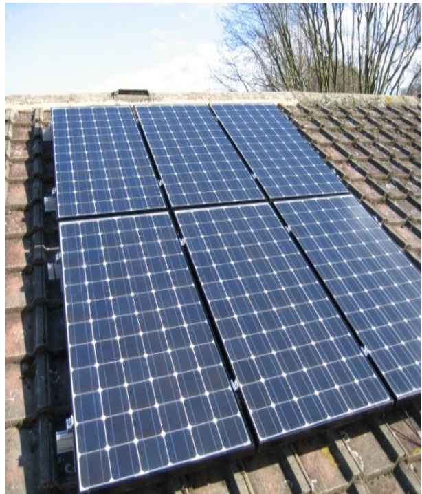
Figure 6 - Photovoltaic array on a pitched roof
