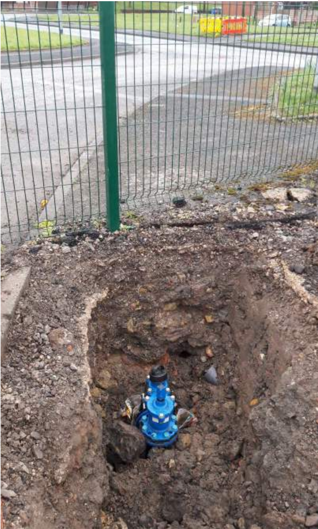
Figure 43 : Washout hydrant used as termination for existing watermain entering site adjacent to Needwood Close gateway
