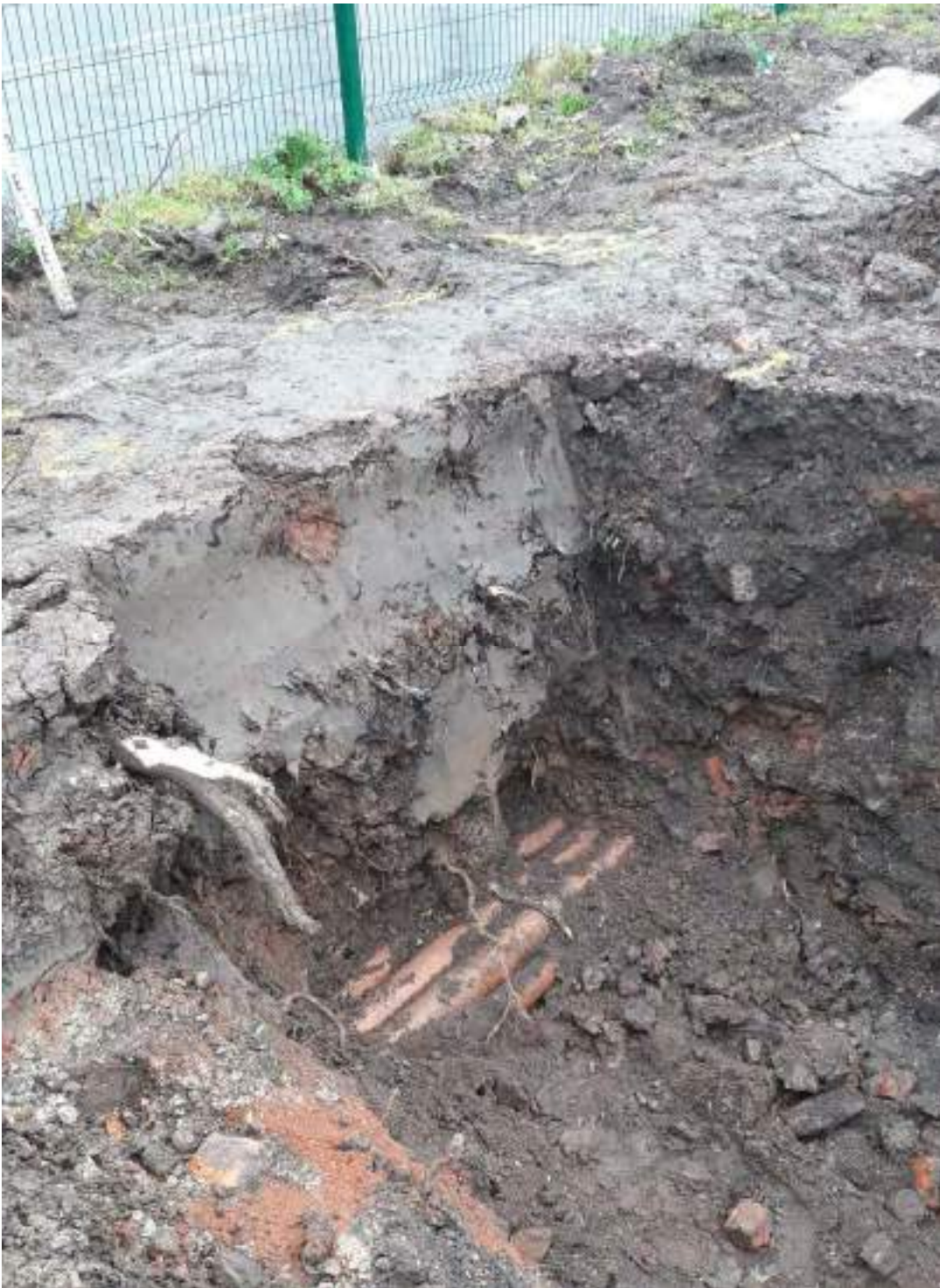
Figure 41 : Seven earthenware BT Openreach ducts located adjacent to Rochdale Road, not relocated
