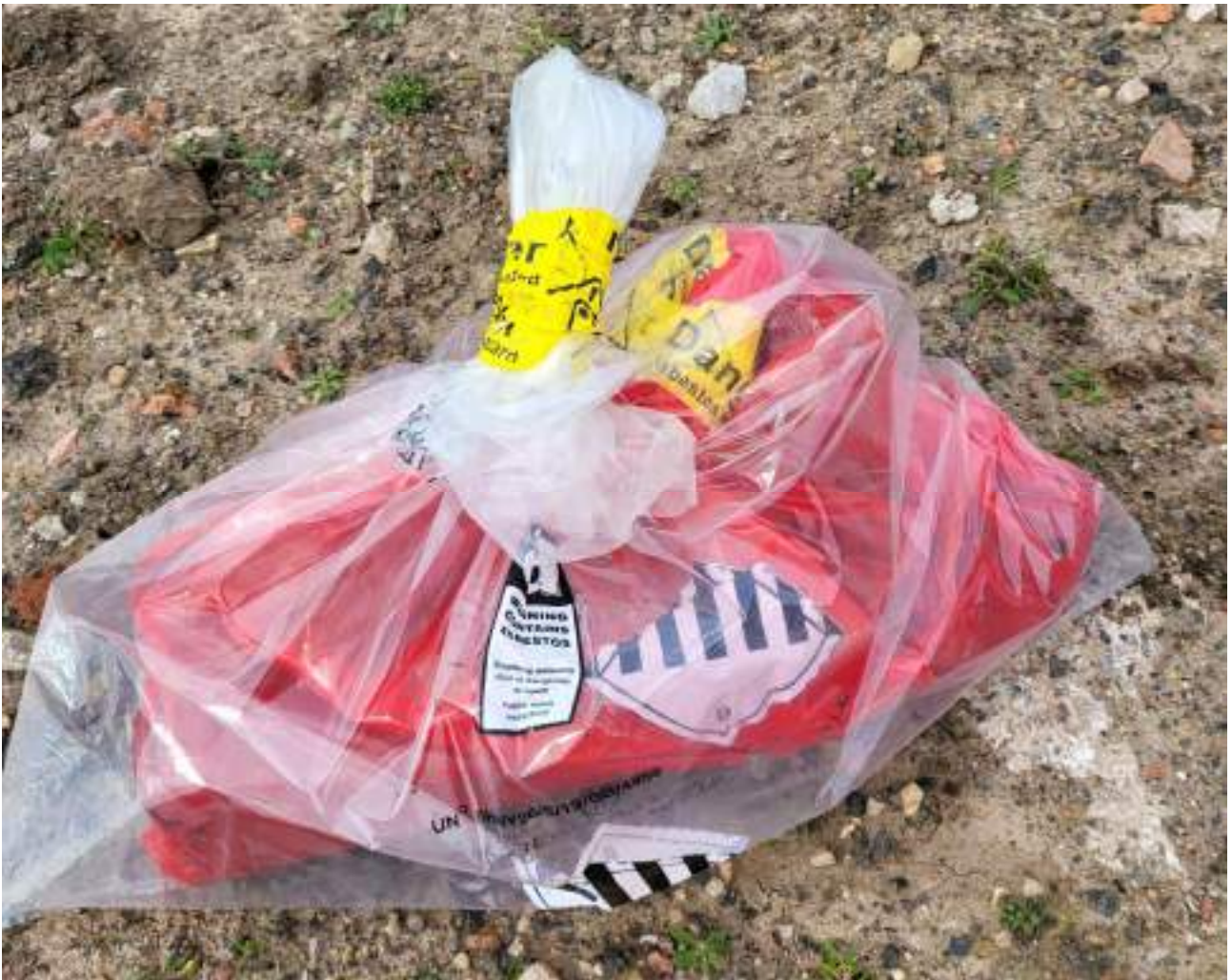
Figure 27 : Pieces of asbestos cement pipe encountered during the works, bagged and awaiting collection by licenced contractor
