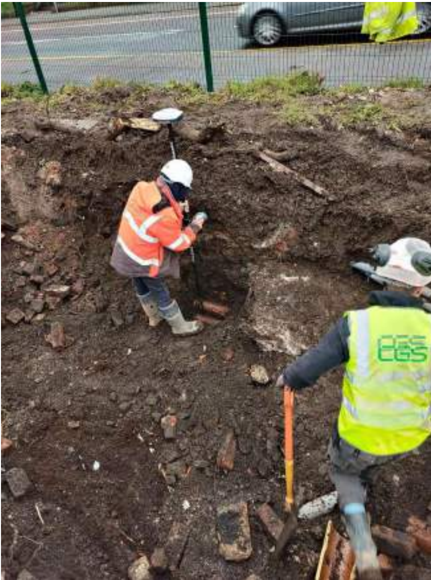
Figure 15 : Concrete obstruction encountered in close proximity to boundary fence and earthenware telecomms ducting
