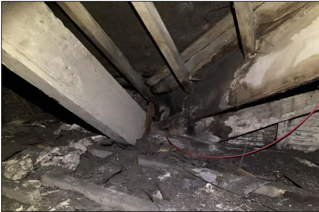
Figure 6 Photograph of roof structure showing water damage.
