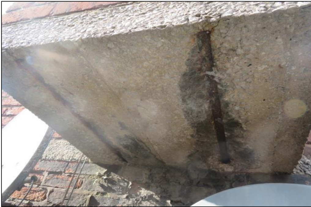
Figure 2: Photograph showing delaminated concrete and spalling brick of the hoist overrun.
