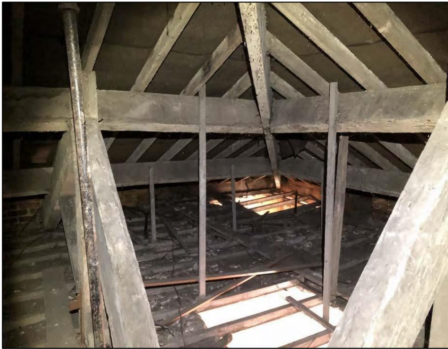
Figure 5: Photograph of roof structure showing extensive deposited 'torching' and failed areas of lath and plaster ceiling.
