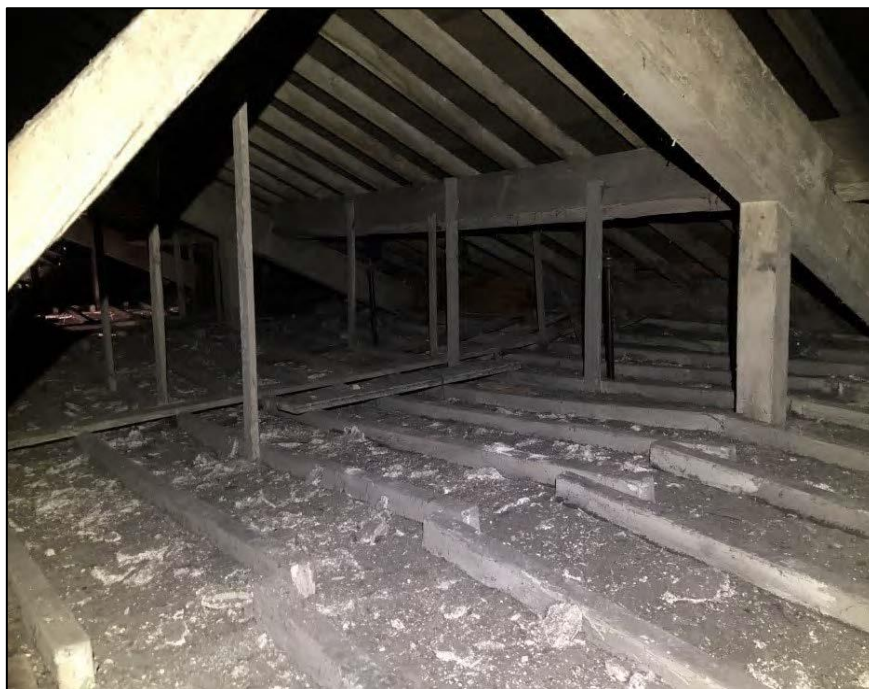
Figure 4: Photograph of roof structure showing extensive deposited 'torching'.
