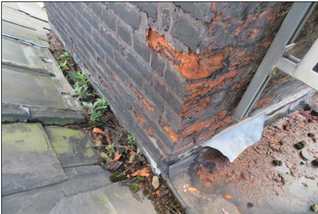
Figure 3: Photograph showing detail of brick shaft with roof valley. The design of which presents an inherent defect vulnerable to failure and build-up of vegetation.
