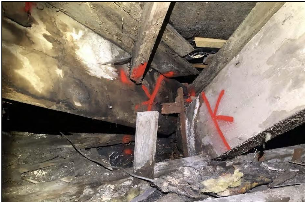
Figure 7: Photograph of roof structure showing water damage.
