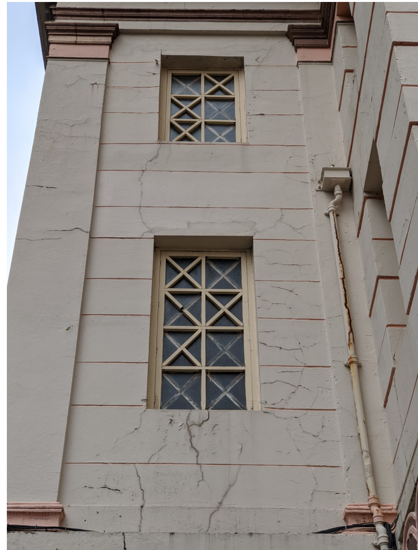
Example of current render condition
