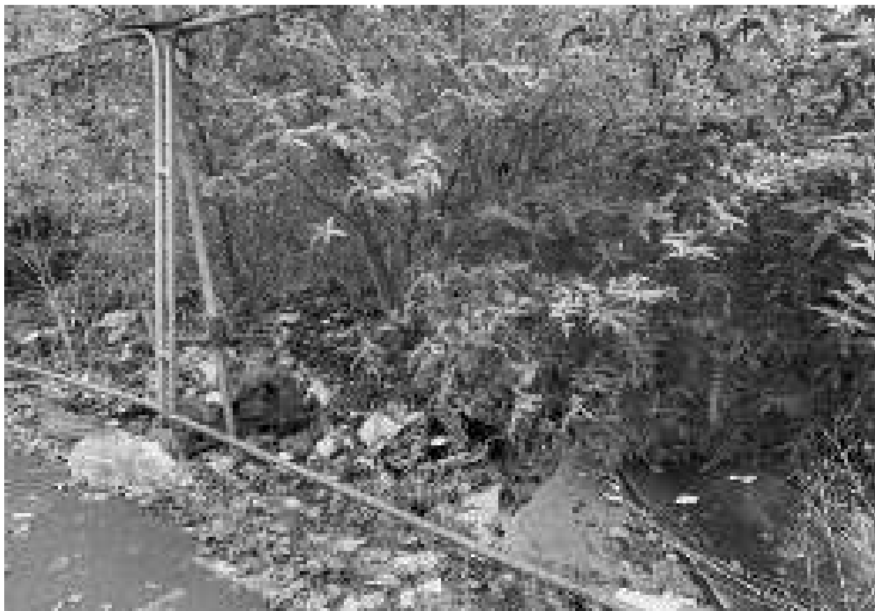
Photograph No 4: Dense Vegetation, Demolition Rubble and Litter
