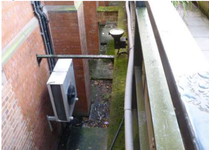
Lightwell to the Rutherford Building, showing Air Handling units that service the stores
