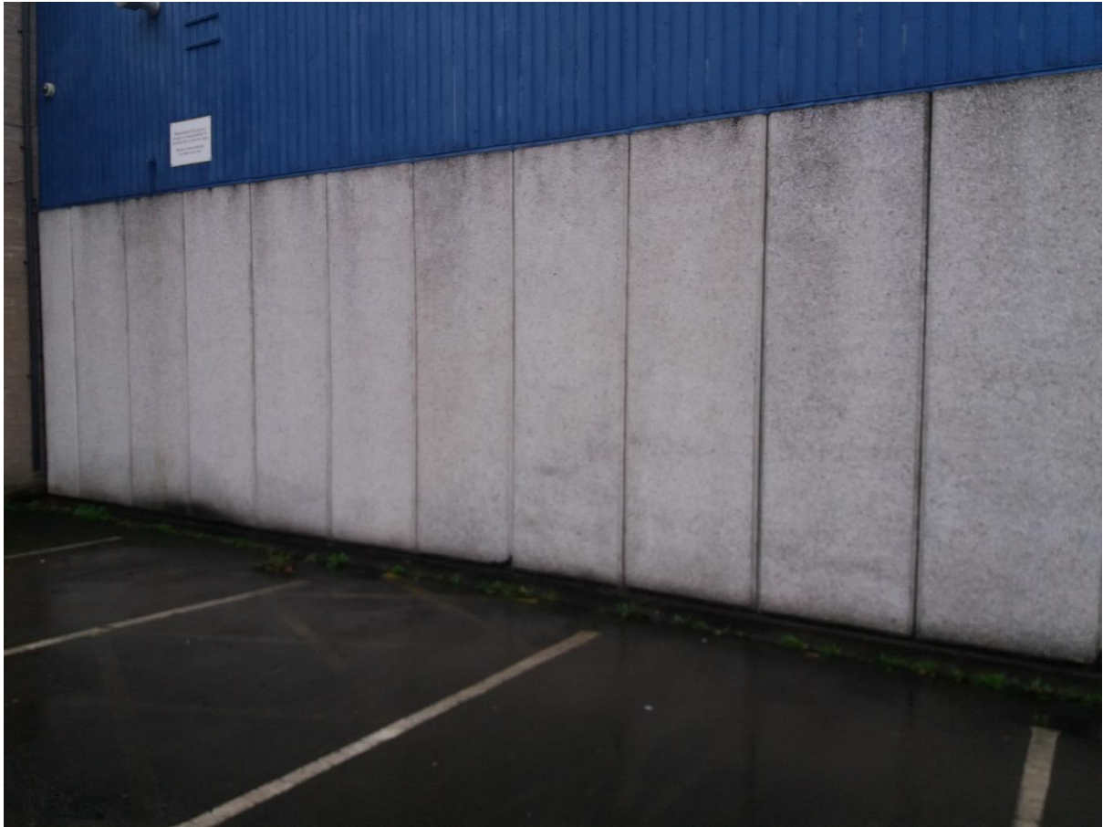
Photo 10: Dirt stained low-level concrete panelling at elevation number 4.
