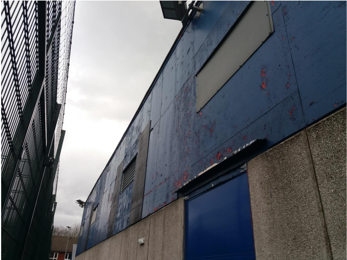
Photo 9: Looking up at elevation number 2. This pic shows the covered ventilation louvers and the poor condition of the flat timber panelling at high level and stained concrete panels at low level.
