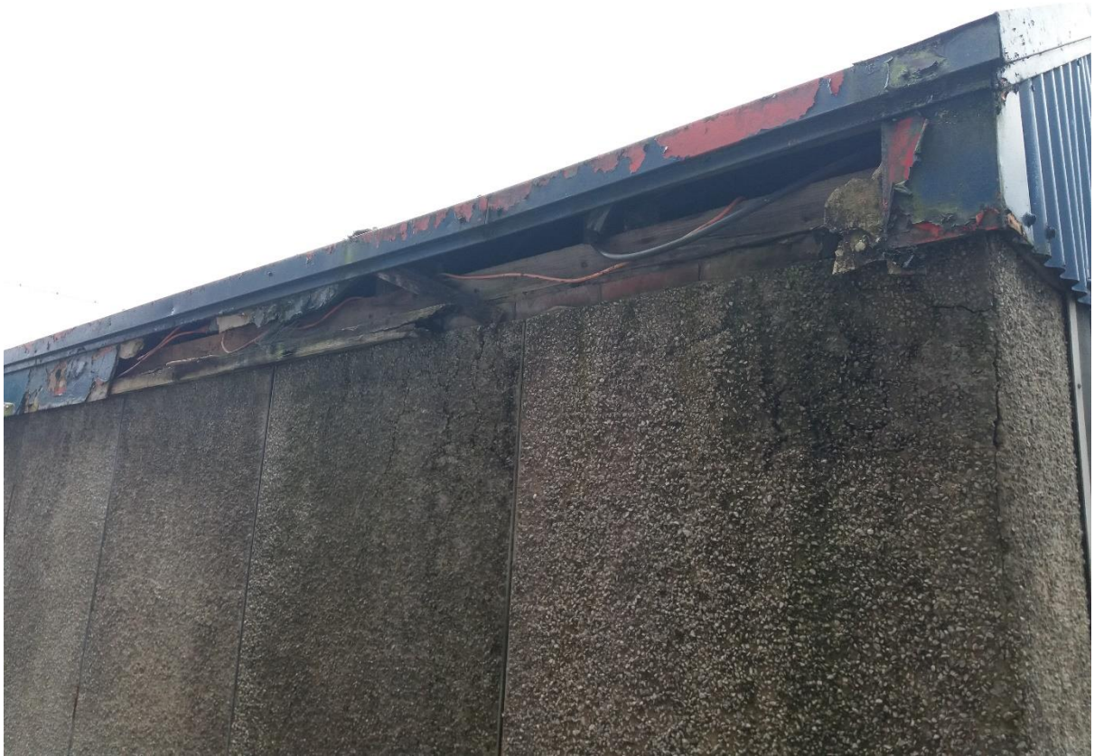
Photo 12: Remains of the existing fascia board to the garage outbuilding.
