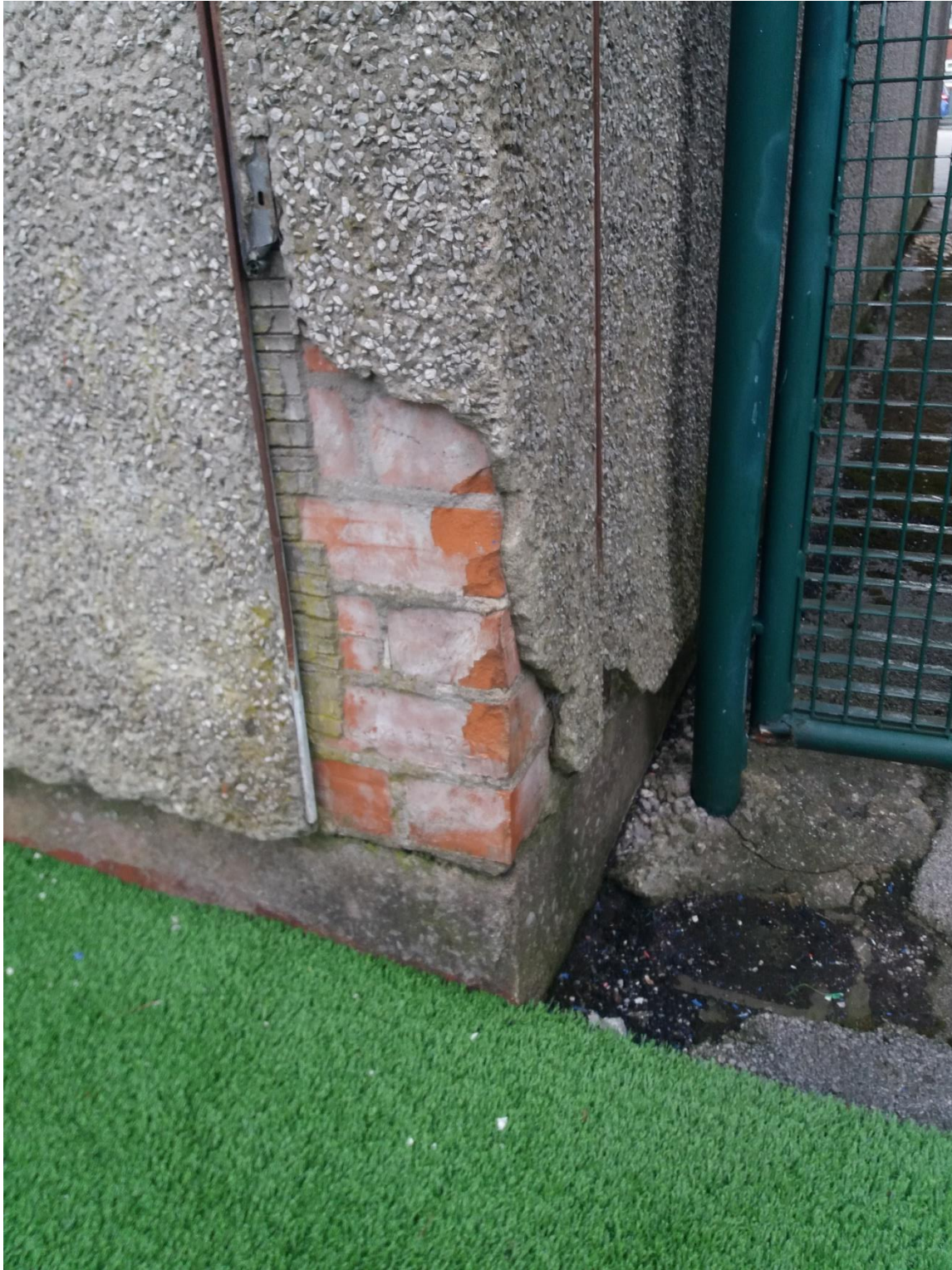
Photo 13: The damaged pebble dashed concrete render to the foot of the wall of the garage outbuilding.
