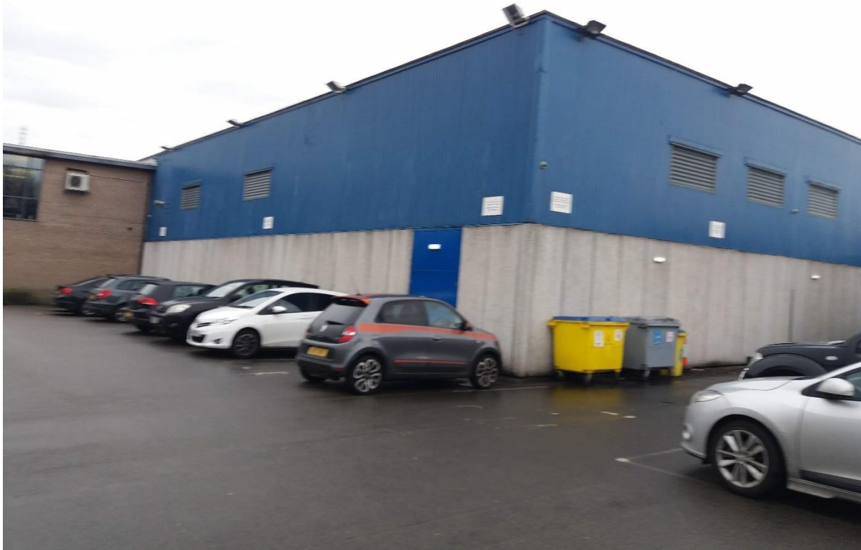
Photo 2: Existing blue coloured high-level timber cladding and low-level concrete cladding panel at the car park elevations. Elevation numbers 3 and 4 on drawing reference ALC-MCC-B01-XX-DR-A-0013.
