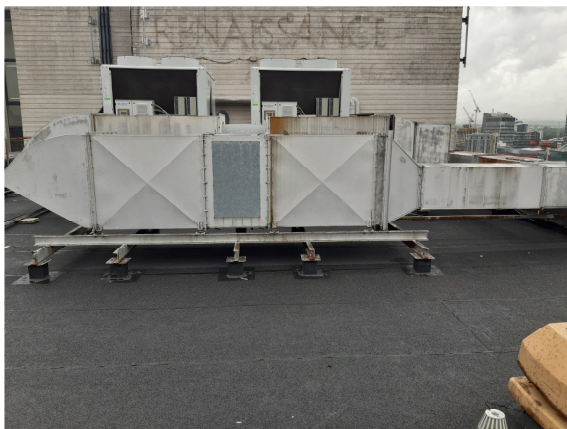
1. Existing roof mounted kitchen ventilation units
