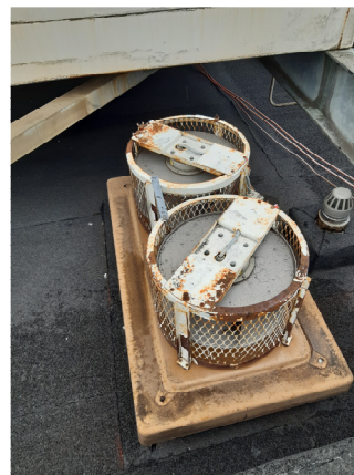
2. Existing roof mounted extract unit serving guest rooms.
