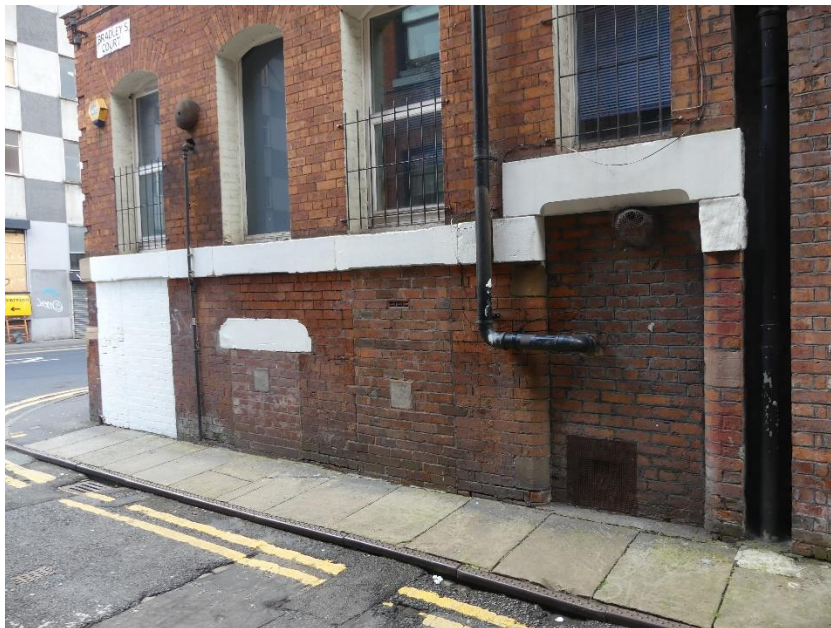
Figure 4.9: The blocked openings to the ground floor to Bradley's Court
