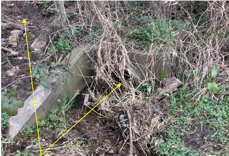
Figure 5: Active drainage discharge into Baguley Brook from other playing pitches via culverts and open ditches (arrowed).
